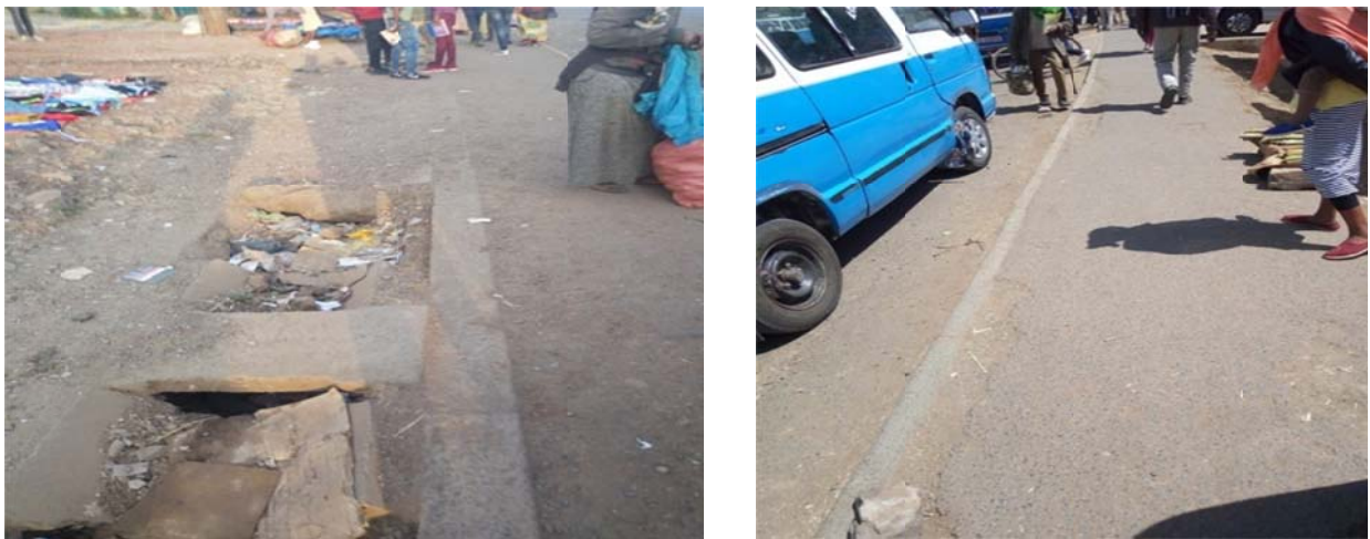
Figure 3-4 : Condition of existing road Around Menagesha
