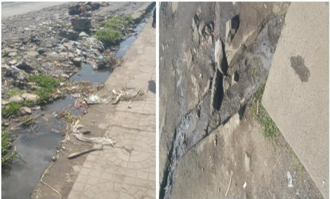
Figure 3: Views of poor drainage network (During site visited 2018).
