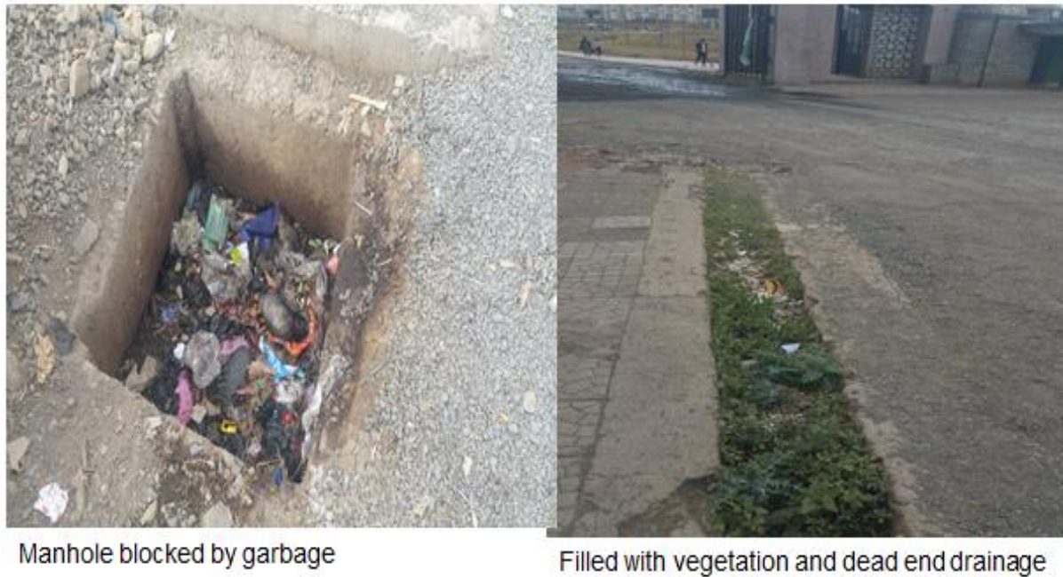
Figure 4 : Conditions of drainage structure. (During site visited 2018).
