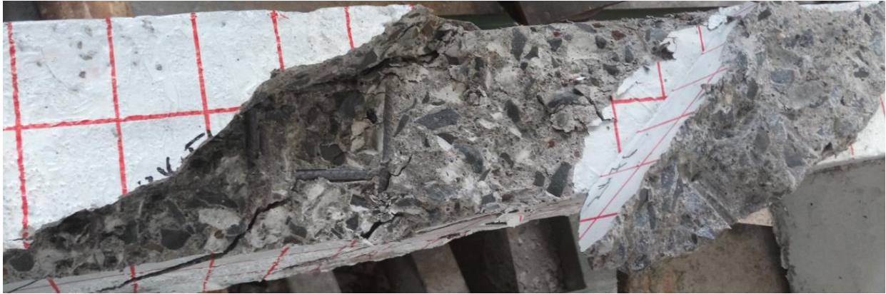
Figure 6-7- Penetrating spiral cracks
