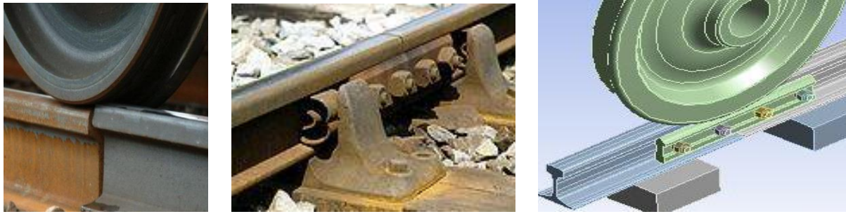
Fig.-5 : Atypical bolt jointed rail
