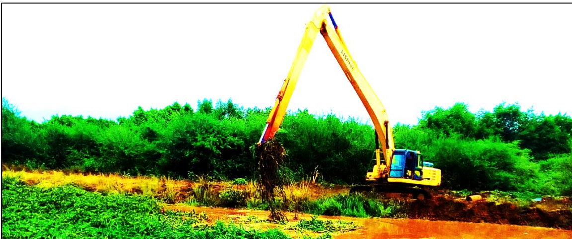
c. Photo of long-armed excavator taken in the Kuraz Irrigation Project(See more in Appendix)
