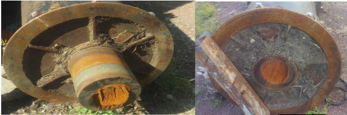
Figure 1.2: Broken existing feeder table head shaft in wonji-shoa sugar factory
