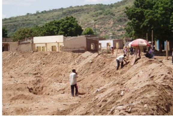
Fig 2.9 Washed out Coca Retaining wall and its vicinity
