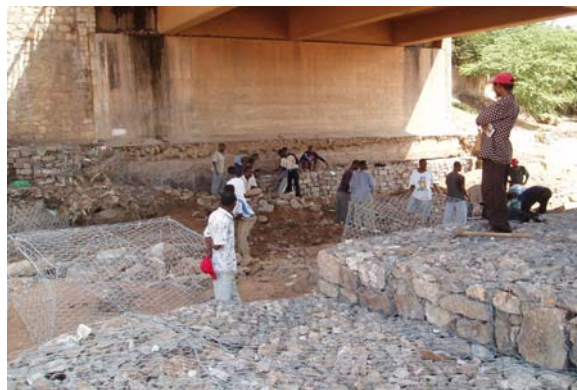
Fig 2.10 Damage Dechatu Main Bridge river bed
