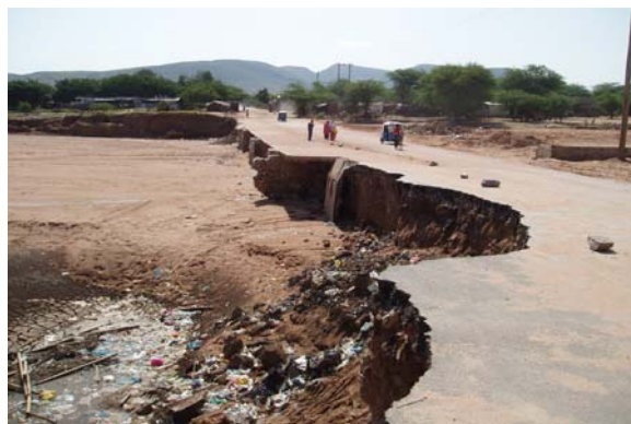
Fig 2.12 Damaged Halfcat crossing
