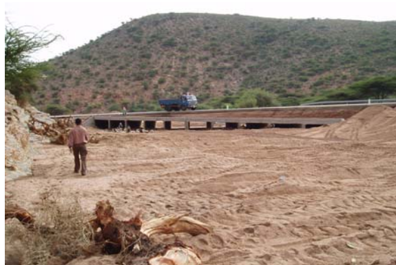
Fig 2.8 Overtopped Menafesha Bridge
