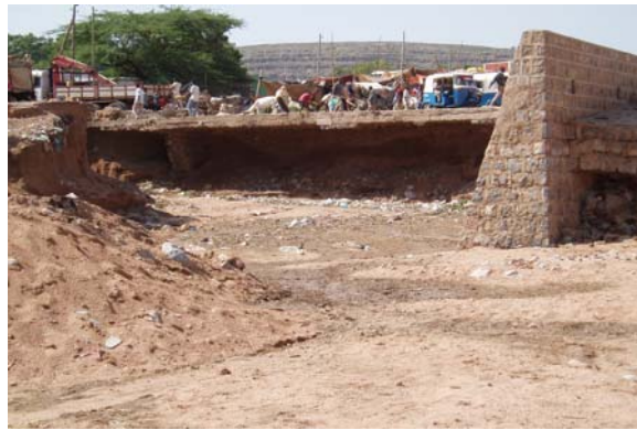
Fig 2.11 Damaged Taiwan Crossing
