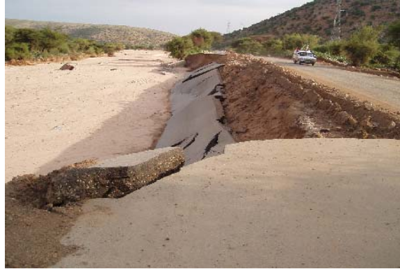
Fig 2.7 Complete Damage of the Main Highway at Hego Village On the main Dengego - Dire Dawa Road by Chirichi River
