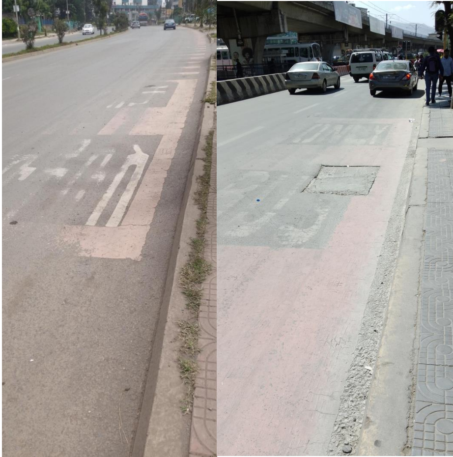
Figure 4.16: Poor lane Marking
