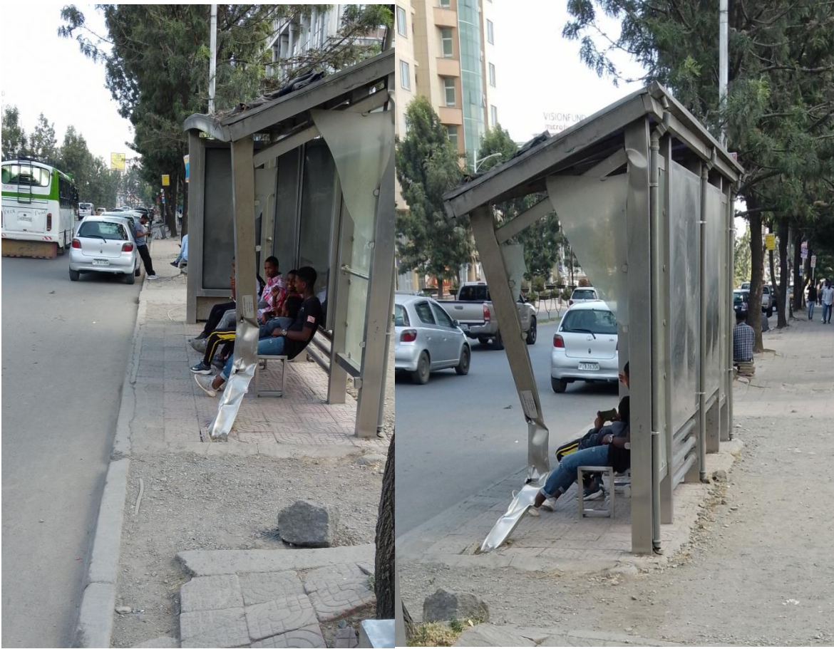
Figure 4.19: Damaged bus stop shelter
