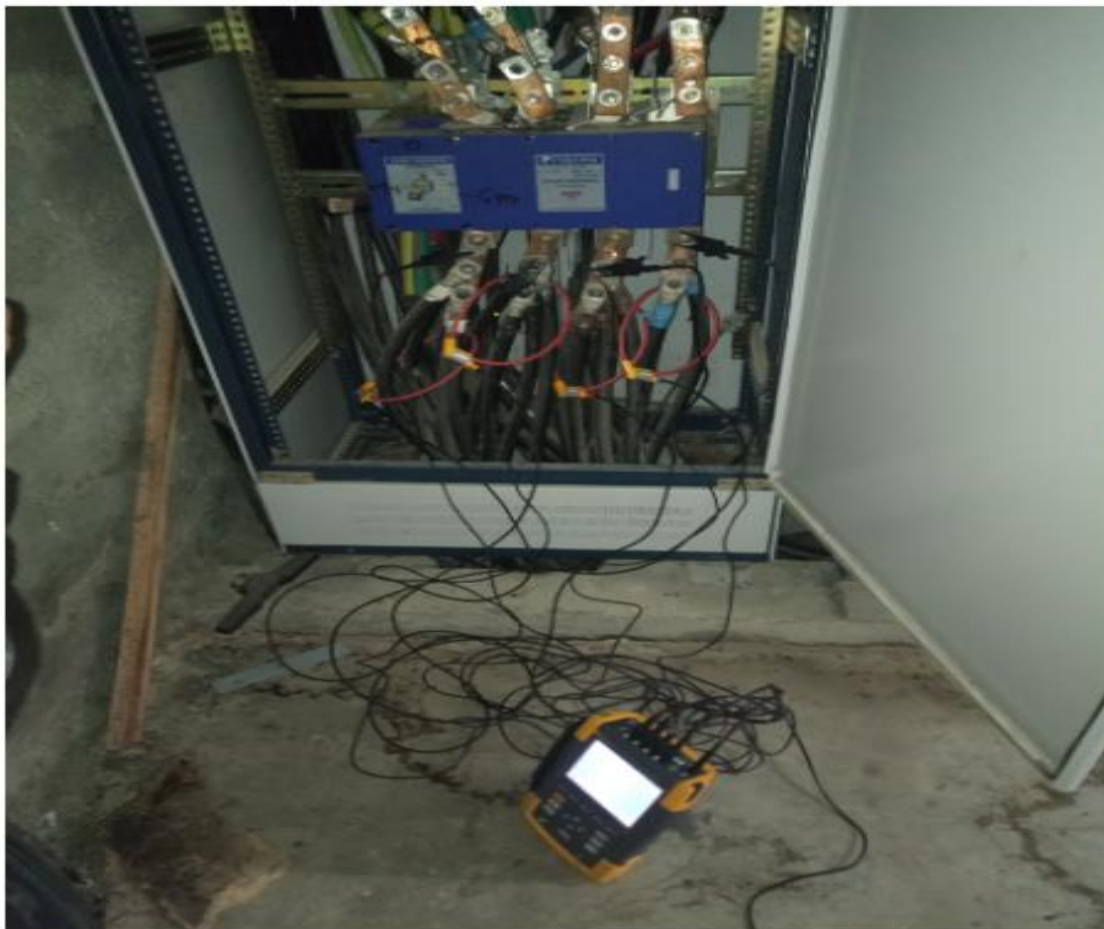
Figure 3-10: The Connection of the Fluke Power Quality and Energy Analyser with the Factory's Transformer during Measurements
