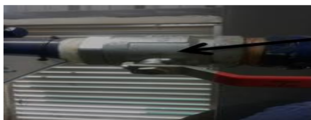
Figure 3-6: Place of Air Leakage Occurred at Air Compressor No-2
