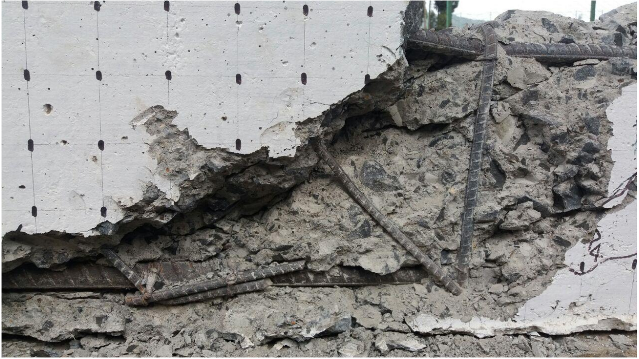
Figure 5-4 Spall concrete cover
