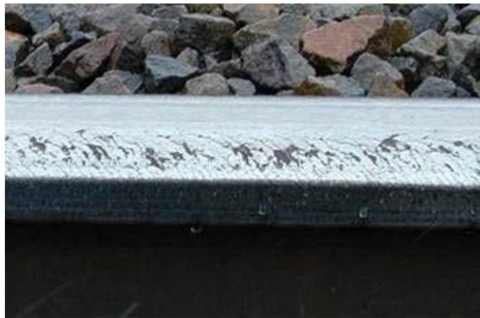
Figure 2.3-3 Sever Head checking
