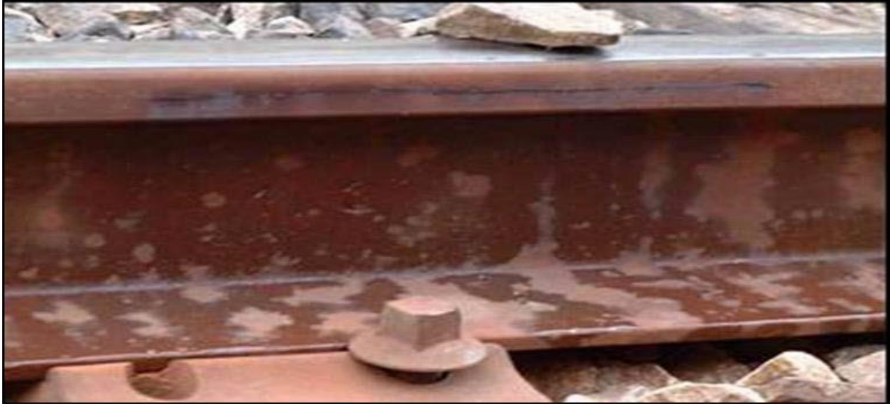
Figure 2.3-2 Progressive horizontal crack
