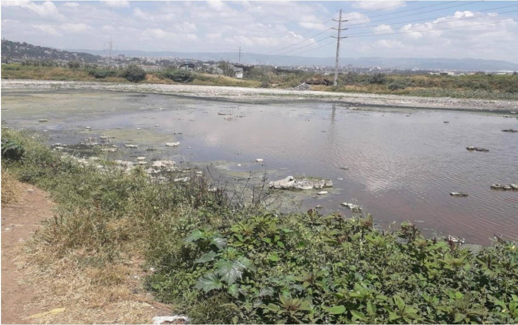
Fig 4.10 Photo shows all city toilet waste sites over flow to village
