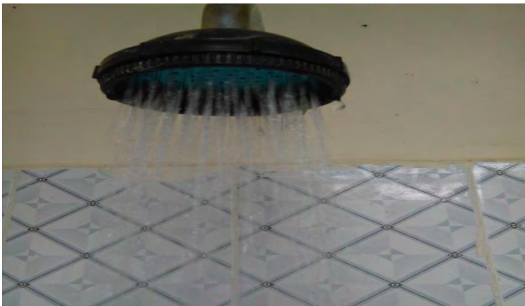
Fig4.3 Shower water becomes hot slowly being opened after a while
