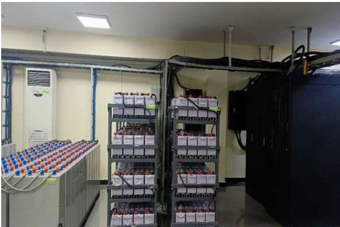
Figure 3.1 Backup battery for Ethio Telecom Microwave Data Center
