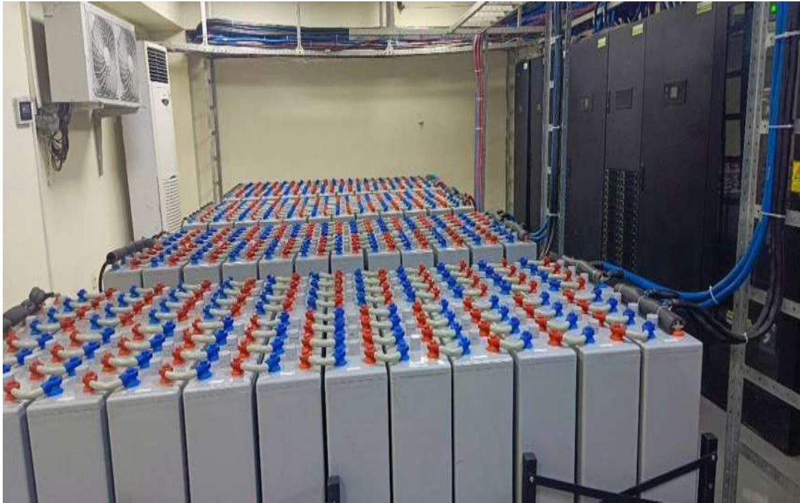
Figure 3.4 Backup battery for Ethio Telecom data center
