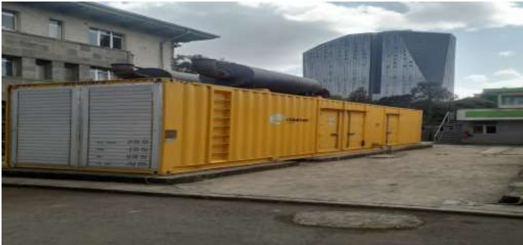
Figure 3.3 Backup Generator for Ethio Telecom Microwave Data Center
