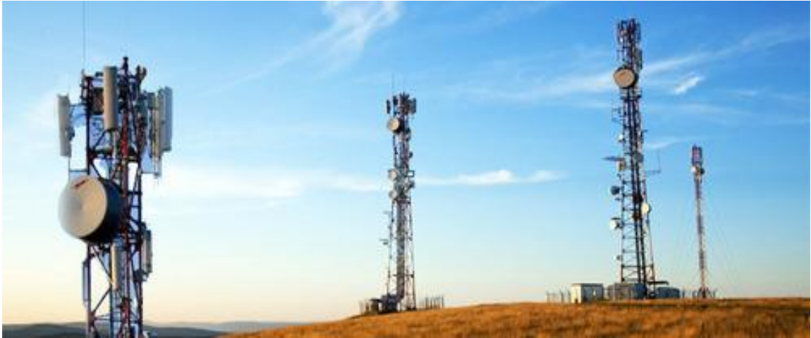
Figure 3. Wireless network tower and antennas
