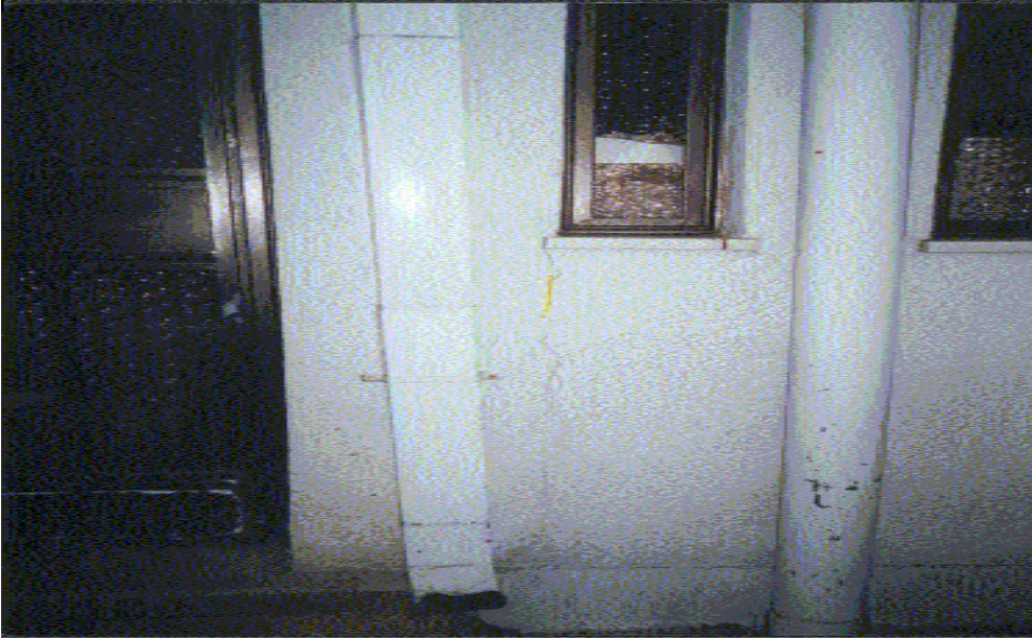
Fig 3.10a Splashing of water to the foundation soil
