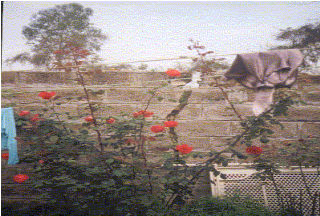
Fig 3.11a Sever vertical crack of fence wall in Mekanisa area .Source of water is from garden watering
