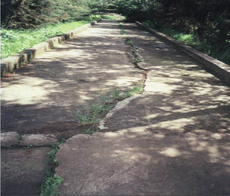
Fig 3.9b Crack of walk way in bole senior secondary school due to lack of void space between the walk way and the concrete curb stone .The source of moisture fluctuation is the surrounding vegetation
