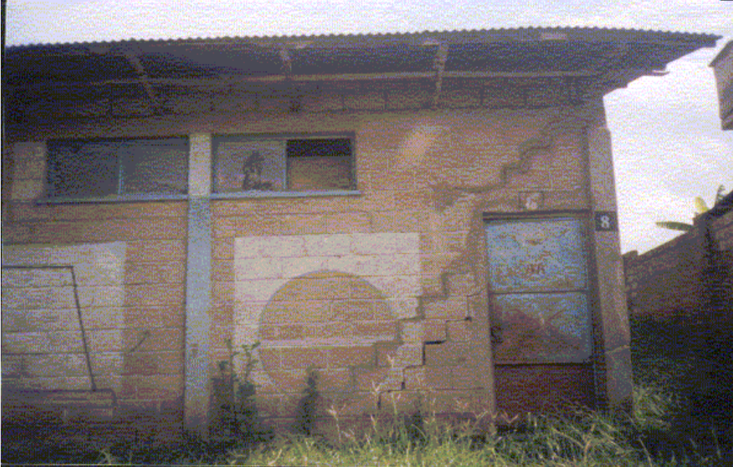
Fig 3.11b Sever diagonal crack of Nesanet public school .The building is surrounded with Shrubs and grasses
