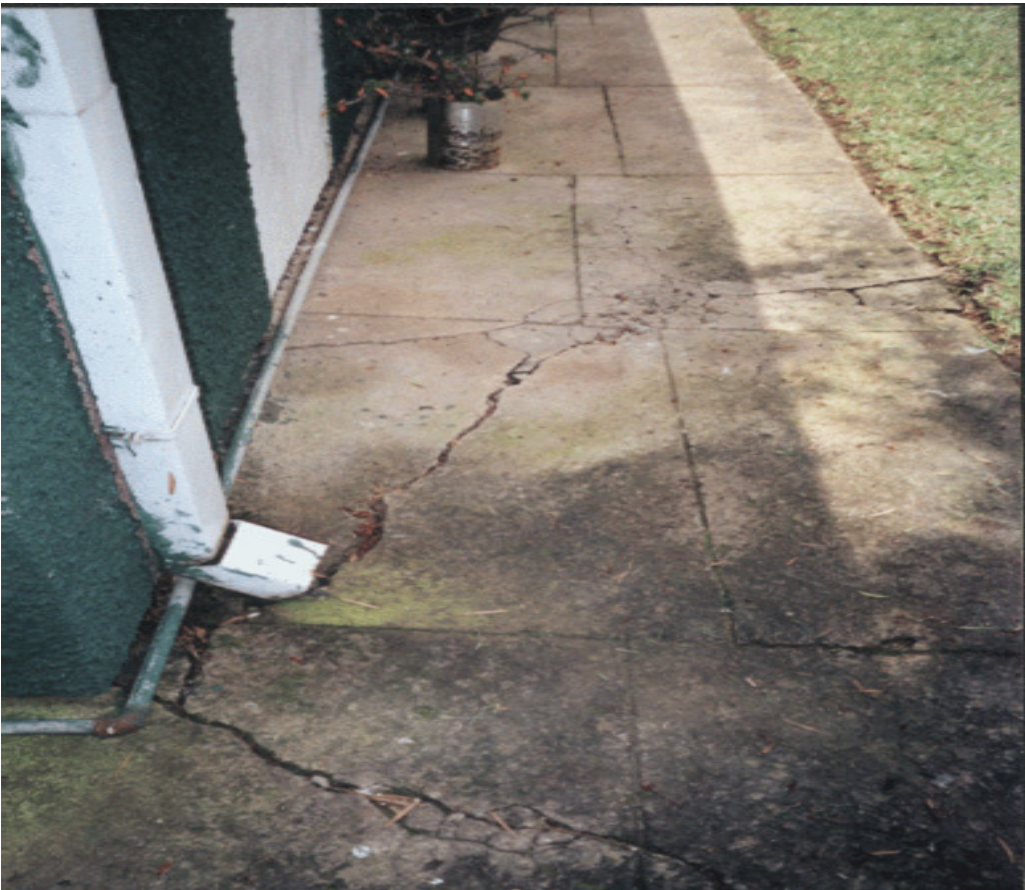
Fig 3.10b leaking of pipe around building and failure of maintaining the down pipe spout
