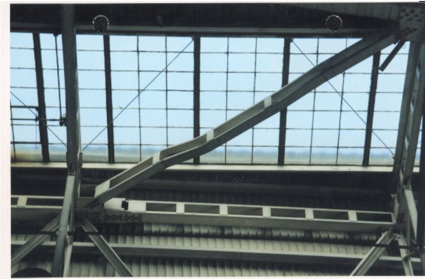
Fig 4.4 Failed truss member of the Ethiopian Airlines maintenance hangar building on Axis-1
