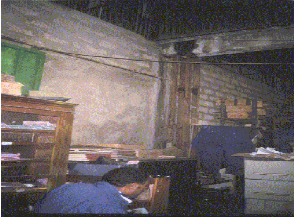
Fig 3.6a Shear of tie beam in Addis Ababa city car maintenance hangar
