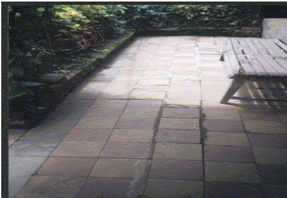
Fig 3.9a Heave of verandah floor in Olympia area due to lack of void between slab and grade beam
