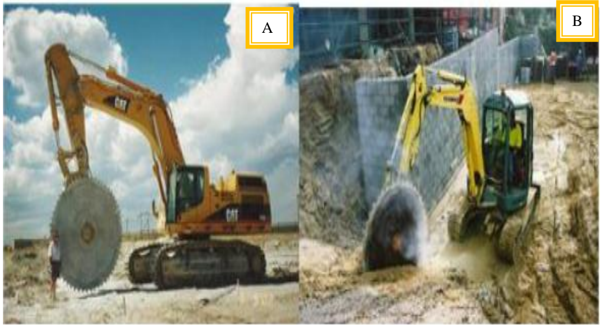
Figure 5.3: A and B, Excavator mounted diamond cutting circular saw is used to produce very large blocks for export.
