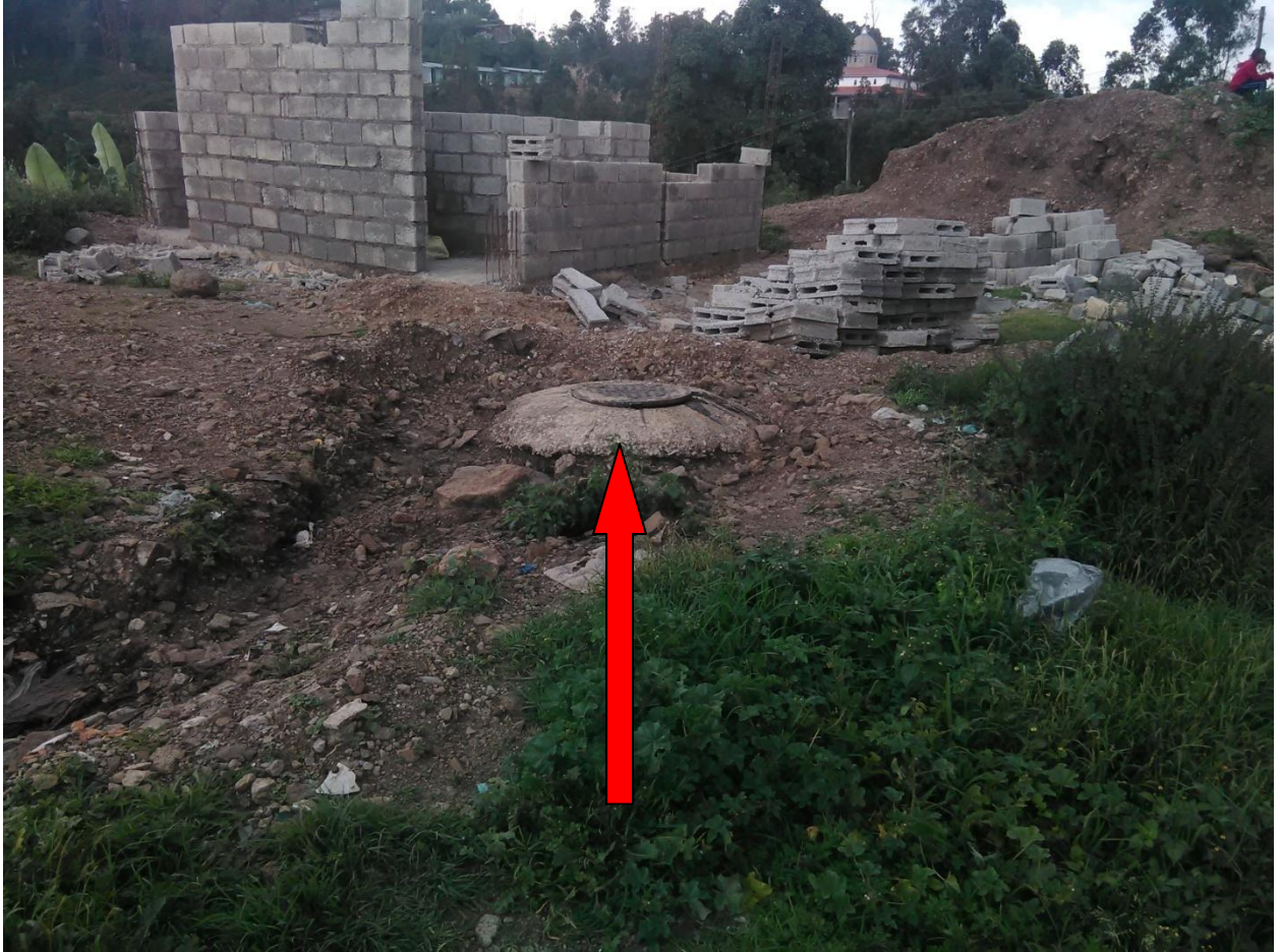
Figure 2. Leaking sewerage (Septic tank), ketena 02, woreda 03, Nefas Silk Lafto Sub-city, Addis Ababa, Ethiopia: 25 September, 2017
