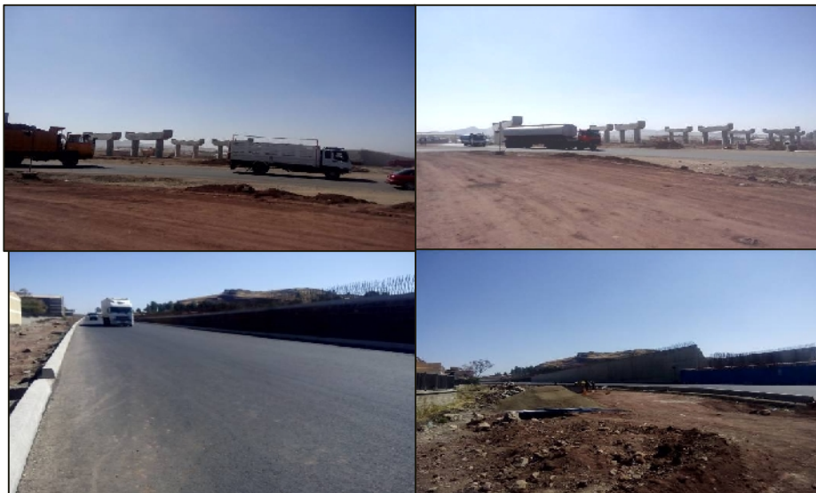
Figure 24: Partial view of the Lebu - Akaki Ring road construction around Tulu Dimtu
