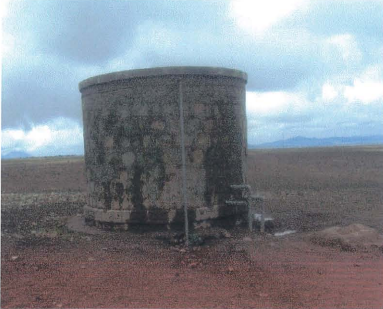
Figure 5-8 Leakage through reservoir located at lowland area
