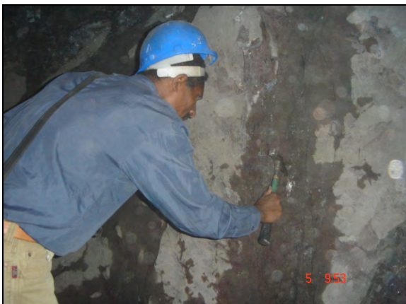
Weathered and fractured breccia basalt on fracture line u/s PH cavern wall
