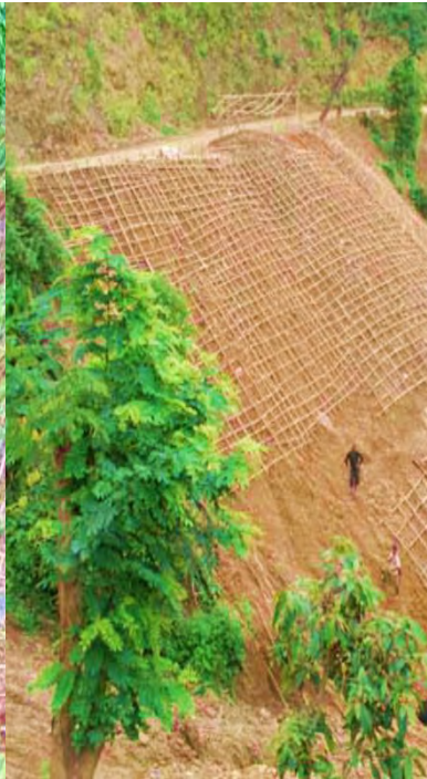
Figure 20: Construction of bamboo knitting structures and the planting of local species of flora in progress
