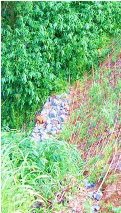
Figure 19: Planting of bamboo over the bamboo structures to complete the process of slope stabilization
