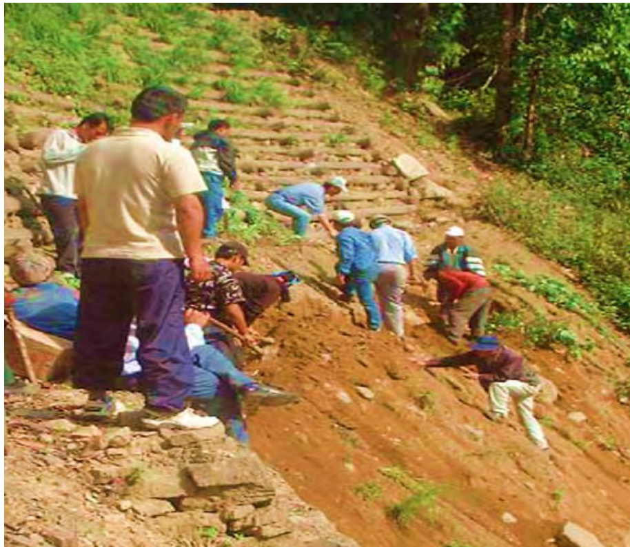
Figure 17: Construction of pine logs to protect the hill slopes under the Bhutan Rural Access Project[24]
