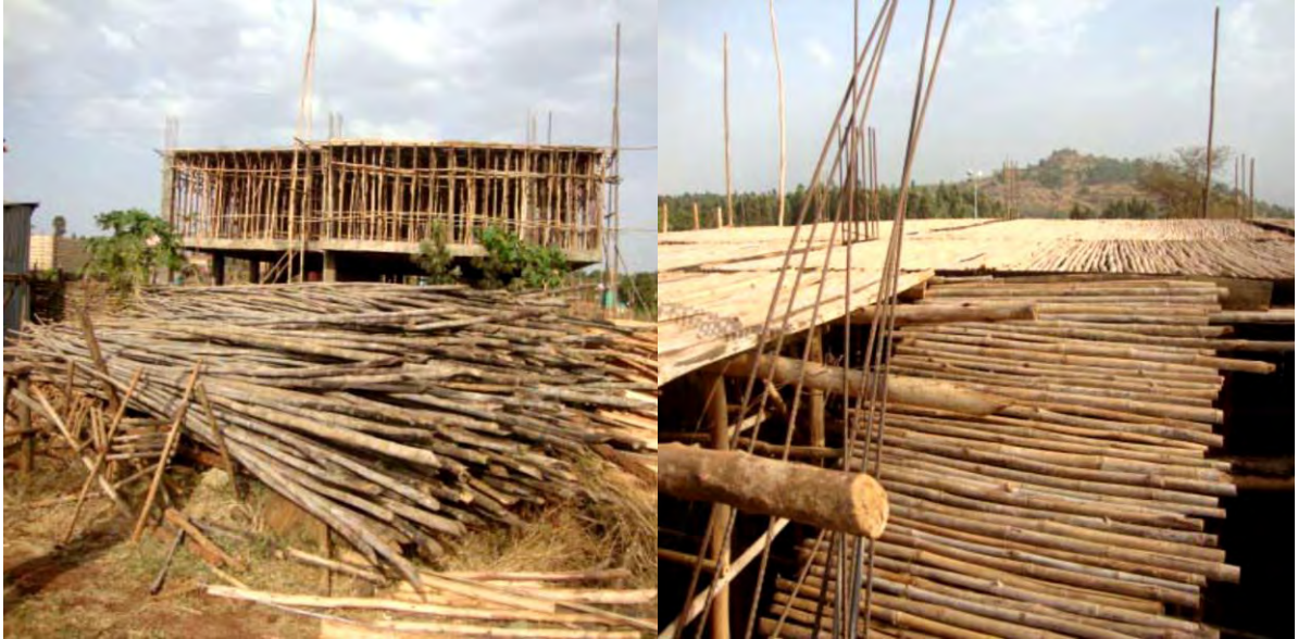
Figure 8: Use of lowland bamboo in scaffolding, and formwork in local flour mills in Assosa town
