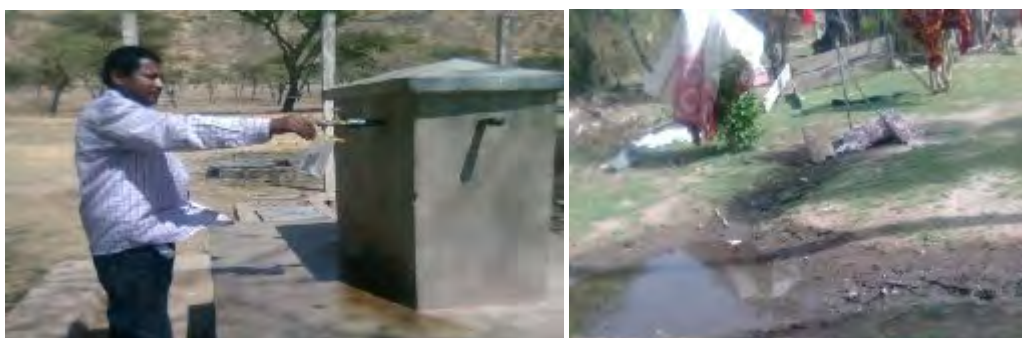
Plate 3.2 sampling and pipe line leakage
