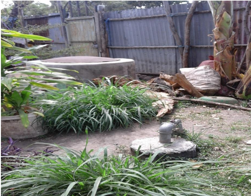
A Biogas digester in the study area
