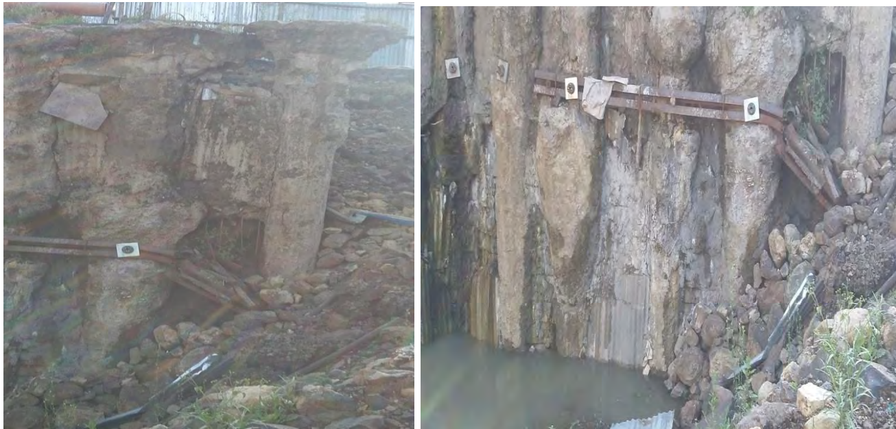
Figure 4.17: Failure of temporary supporting piles including the anchor
