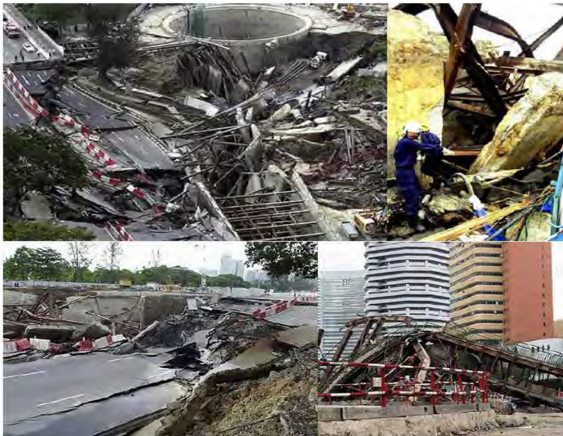
Figure 2.9:- Mass Rapid Transit cut and cover excavation failure – Singapore [9]
