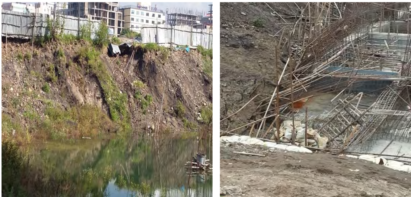
Figure 4.7: Lack of protection wall & sliding of the ground results collapse of the fence
