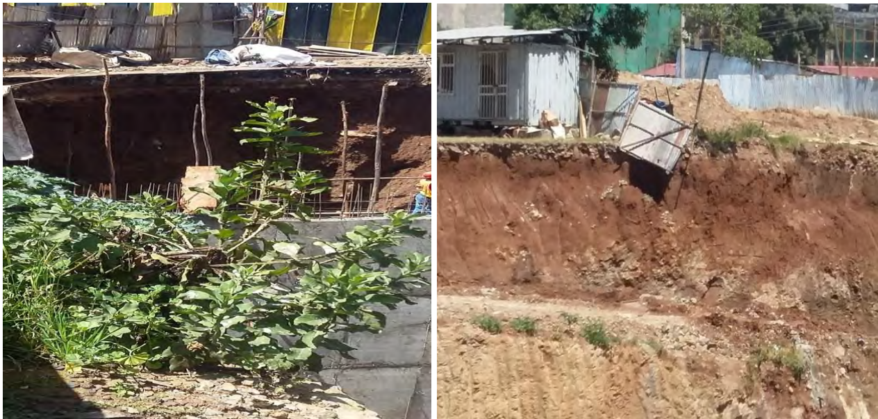
Figure 4.10: (B) Sliding & collapse of structure due to wrong calculation of earth pressure
