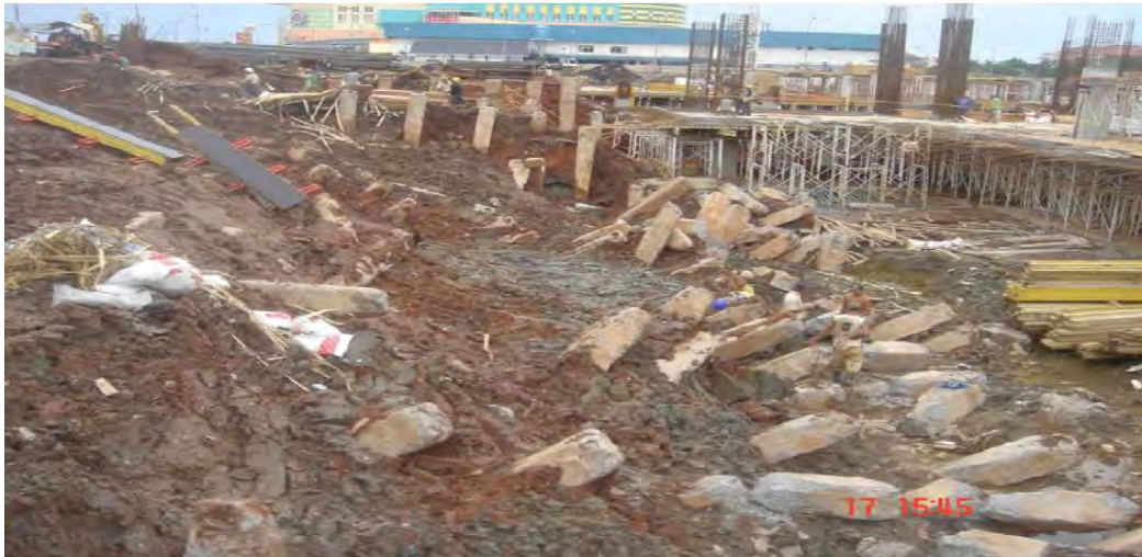
Figure 2.5:- Failure of Open cut Excavation that Lead to Driven Pile Foundation Failures- North Jakarta-2005 [9]
