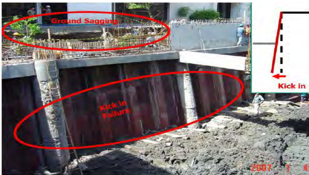
Figure 2.6:- Kick in Failure of Sheet Pile-Surabaya-2007
