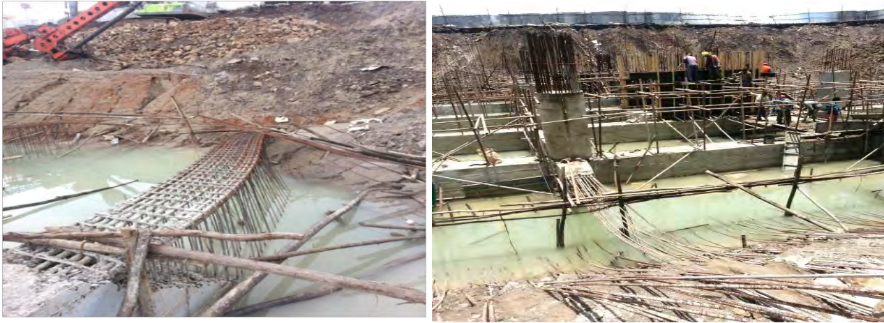
Figure 4.14: Deformation of re-bars due to sliding of the ground & presence of ground water
