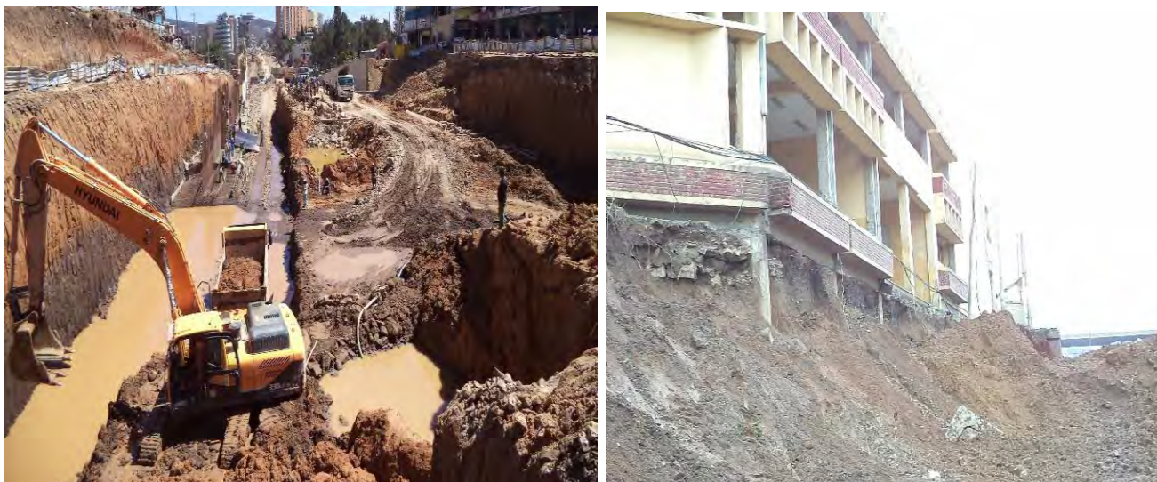
Figure 4.8: Practice of AALRT projects; lack of dewatering & protection nearby structure
