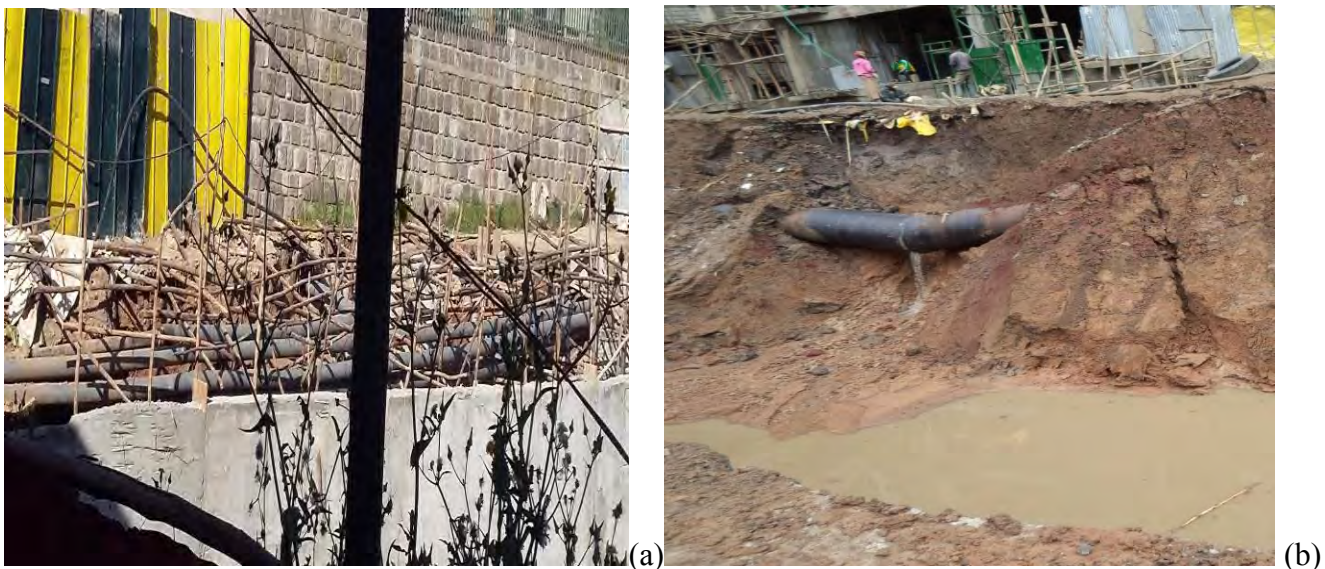
Figure 4.11: Sliding effect on utility lines and the sliding results unsafety environment neighborings
