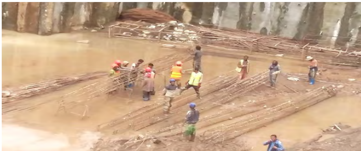
Figure 4.4:- Unsafe & inappropriate working condition; poor reinforcement placement
