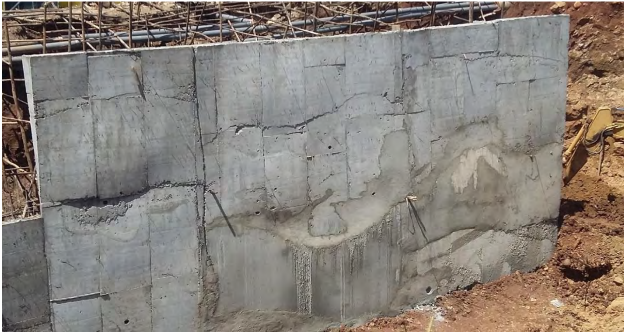
Figure 4.19: Poor quality of concrete retaining wall, improper erection of formwork results deformed structure
