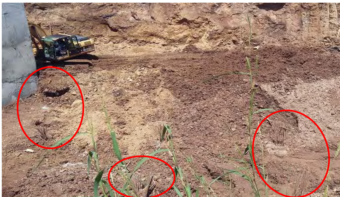
Figure 4.9: Wrong calculation of soil pressure results in sliding & failure of foundation
