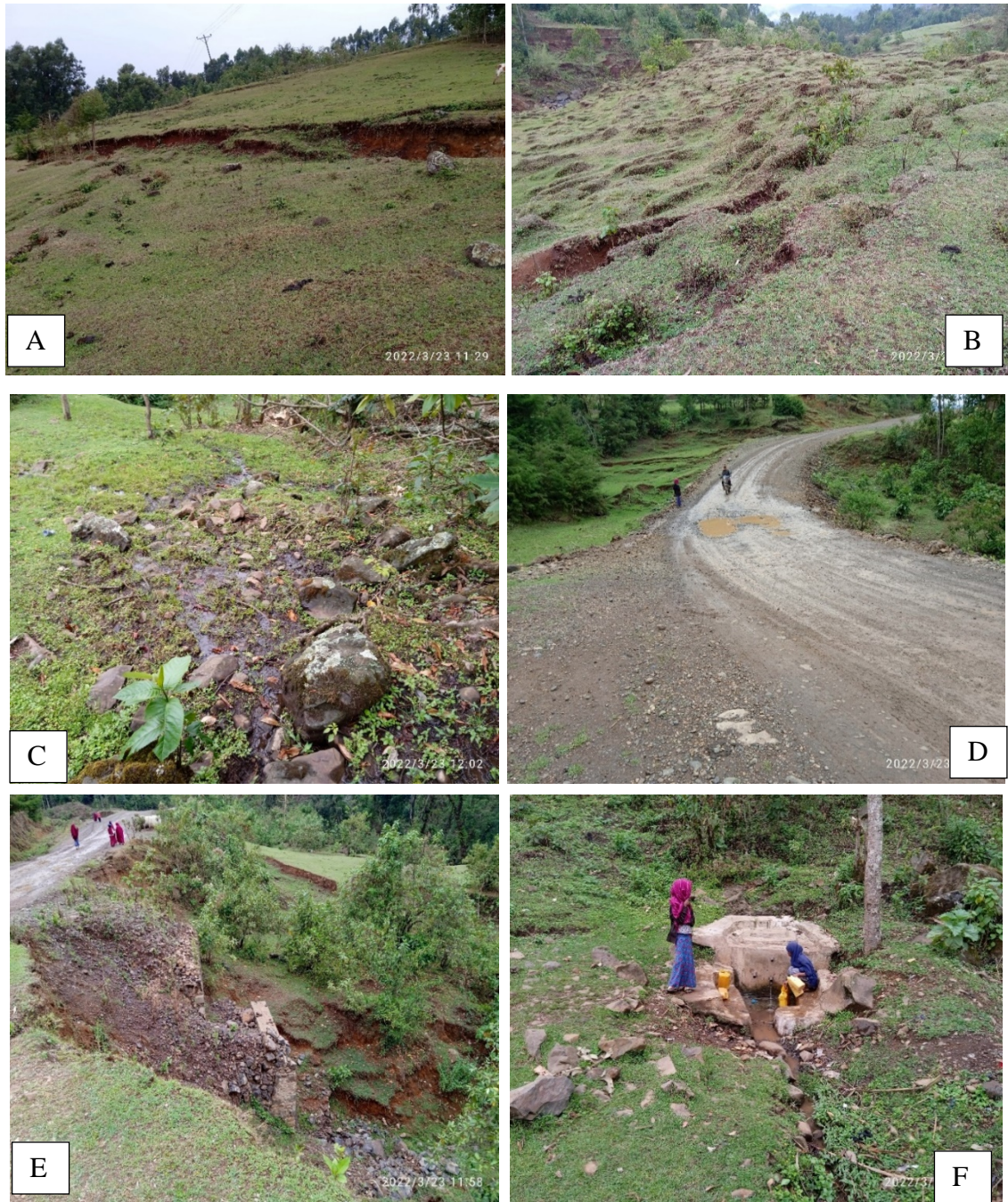
Plate 4-5: Landslide at site JC/S/05: A) Main scarp on the back slope B) Severely destabilized area of the river bank on the upstream C) Swampy area due to springs D) Sag on the existing road due to movement E) Failed drainage structure F) Water well developed from the spring indicating the presence of sub-surface water at shallow depth.
