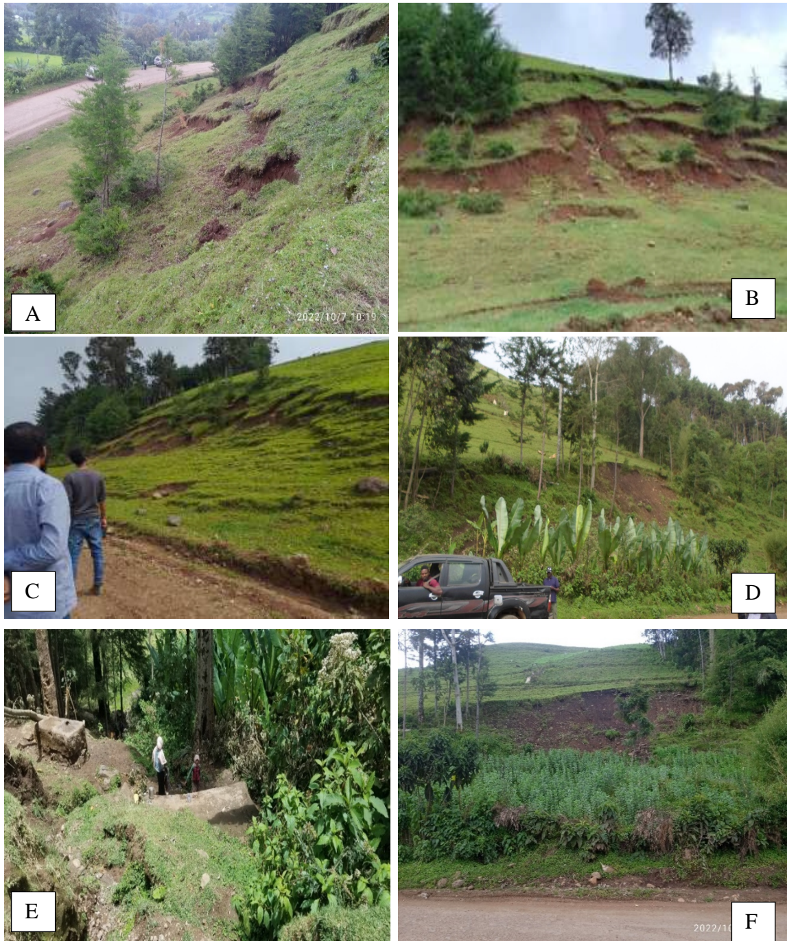
Plate 4-2: Landslide at site JC/S/02; A-C Slope movement of the brownish, loose silty clay soil with gravel at the back slope of the road D) Landslide at the back slope of the road E) Developed water well on the left side of the road indicating the presence of ground water at shallow depth F) Landslide of the back slope with prominent semi-circular scarp.
