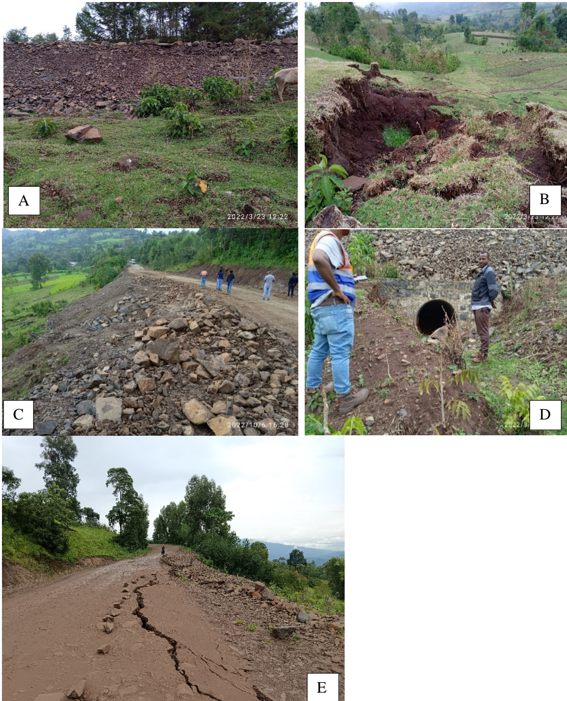
Plate 4-7: Landslide at site JC/S/07: A)Backfilled material on the failed section B)Mobilized mass at the toe of the landslide C)Landslide from the side slope direction of the road D)Clogged cross drainage ditch on the downstream E)Main scarp on the road surface re-emerge on the July 31,2023.
