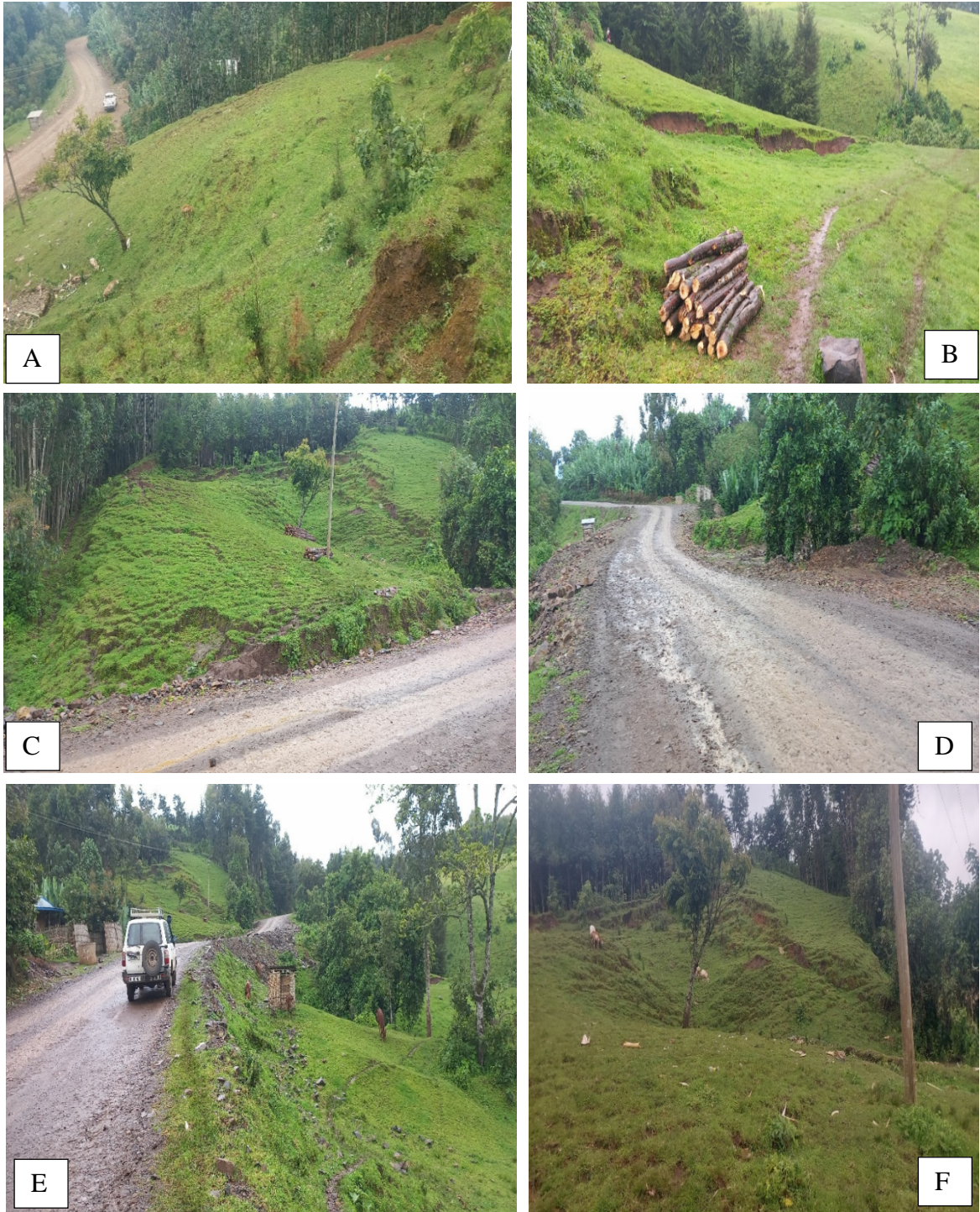
Plate 4-3: Landslide at site JC/S/03 A) Landslide from the top of the scarp) Crack on the left flank of the landslide extended to the side slope C) Depleted mass on the back slope side of the road D) The gravel wearing road near the failed section (toward Chida) E) Potentially unstable area near the active landslide F) Depletion on the back slope of the slide mass.
