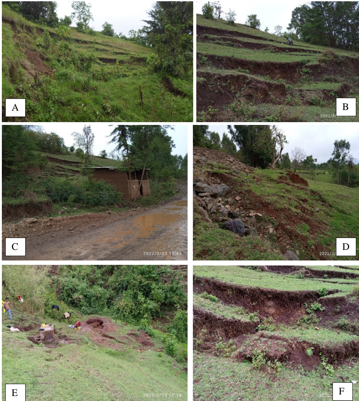
Plate 4-8: Landslide at site JC/S/08 A)Landslide on the back slope of the road B) Multiple tension cracks on the slope C)House constructed on the sliding mass D)Destabilized mass on the side slope of the road E)Wet/swamp area at the toe of the side slope due to multiple springs F)Big tension cracks on main scarp on the top of the landslide.
