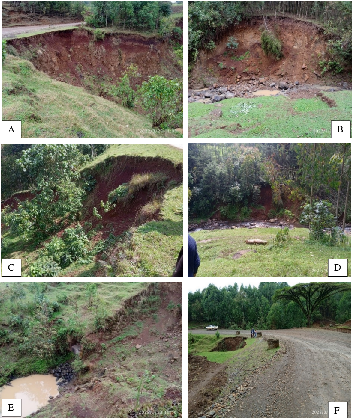
Plate 4-4: Landslide at site JC/S/04 A)Severe erosion propagated to landslide B)Erosion of river bank on the downstream direction C)Localized old landslide propagating towards the road D)Erosion of the river bank on upstream side E)Toe erosion of the side slope by the water from the drainage outlet F)Land slide initiated by severe erosion propagating to the road.
