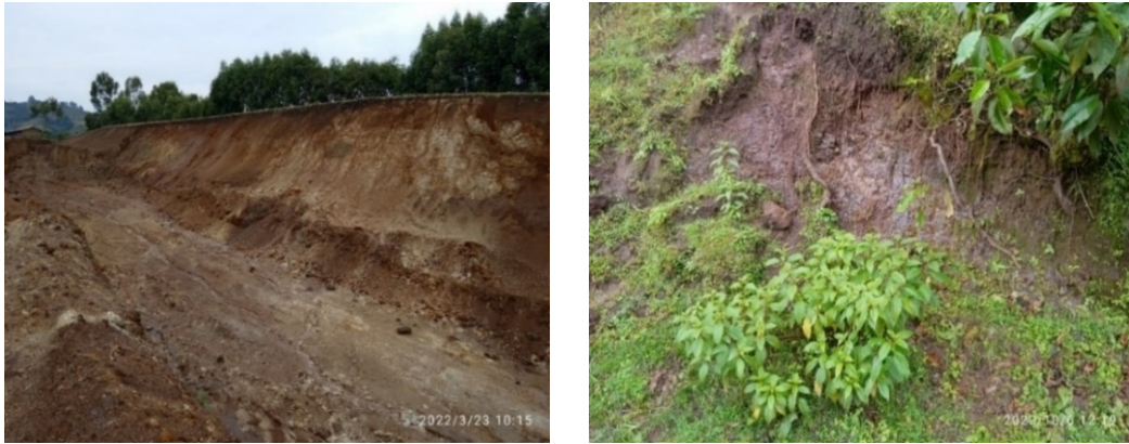
Figure 3-8: Highly weathered to decomposed rock along Jimma-Chida road section with relict structures and fabric still preserved
