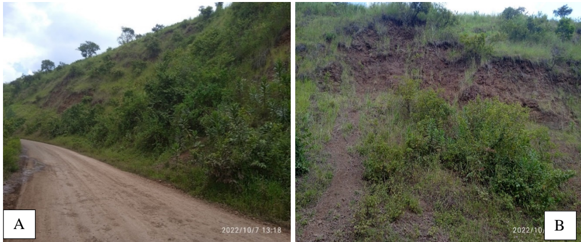
Plate 4-10: Landslide at site JC/S/10: A)Steep back slope with low severity rock fall and minor slide B)The exposed, highly weathered and fractured slope material.
