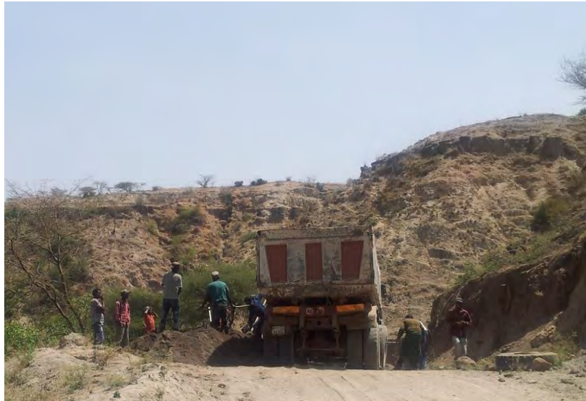
Figure 14 Sand loading to a dump truck from a vehicle accessible place in site B (picture taken by researcher).
