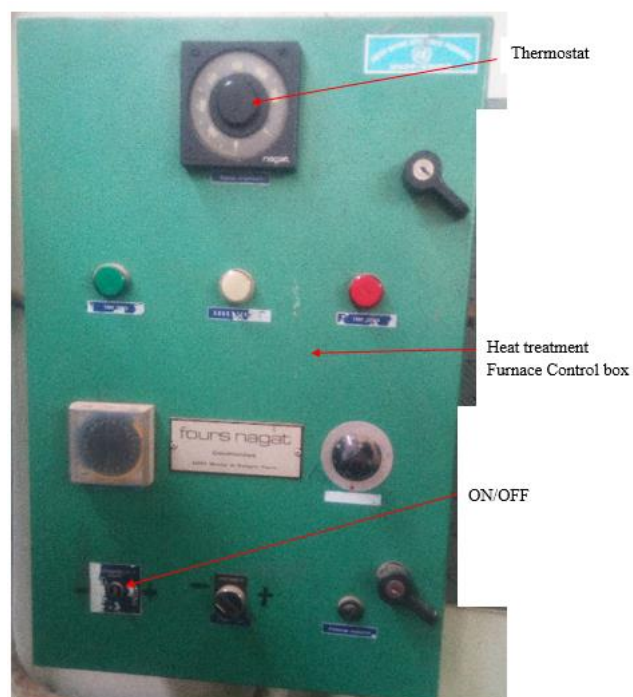
Figure 3.4 Heat treatment furnaces temperature control box
