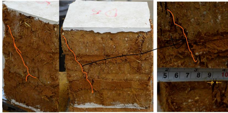
Figure 4-16 crack pattern and crack width of specimen D5
