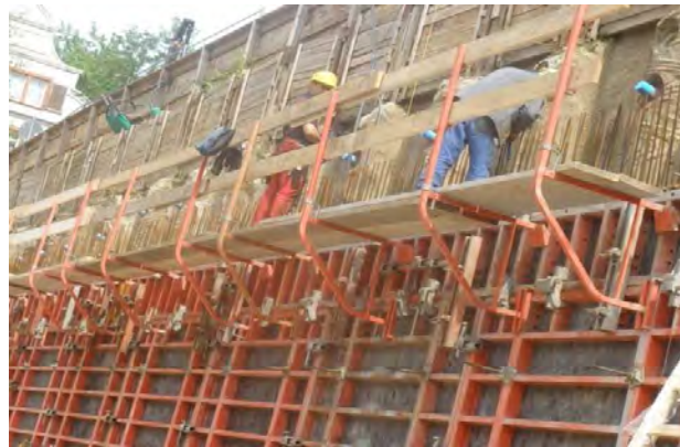
Figure 4.7 Safety Guard Rails and Platform, Darmstadt
