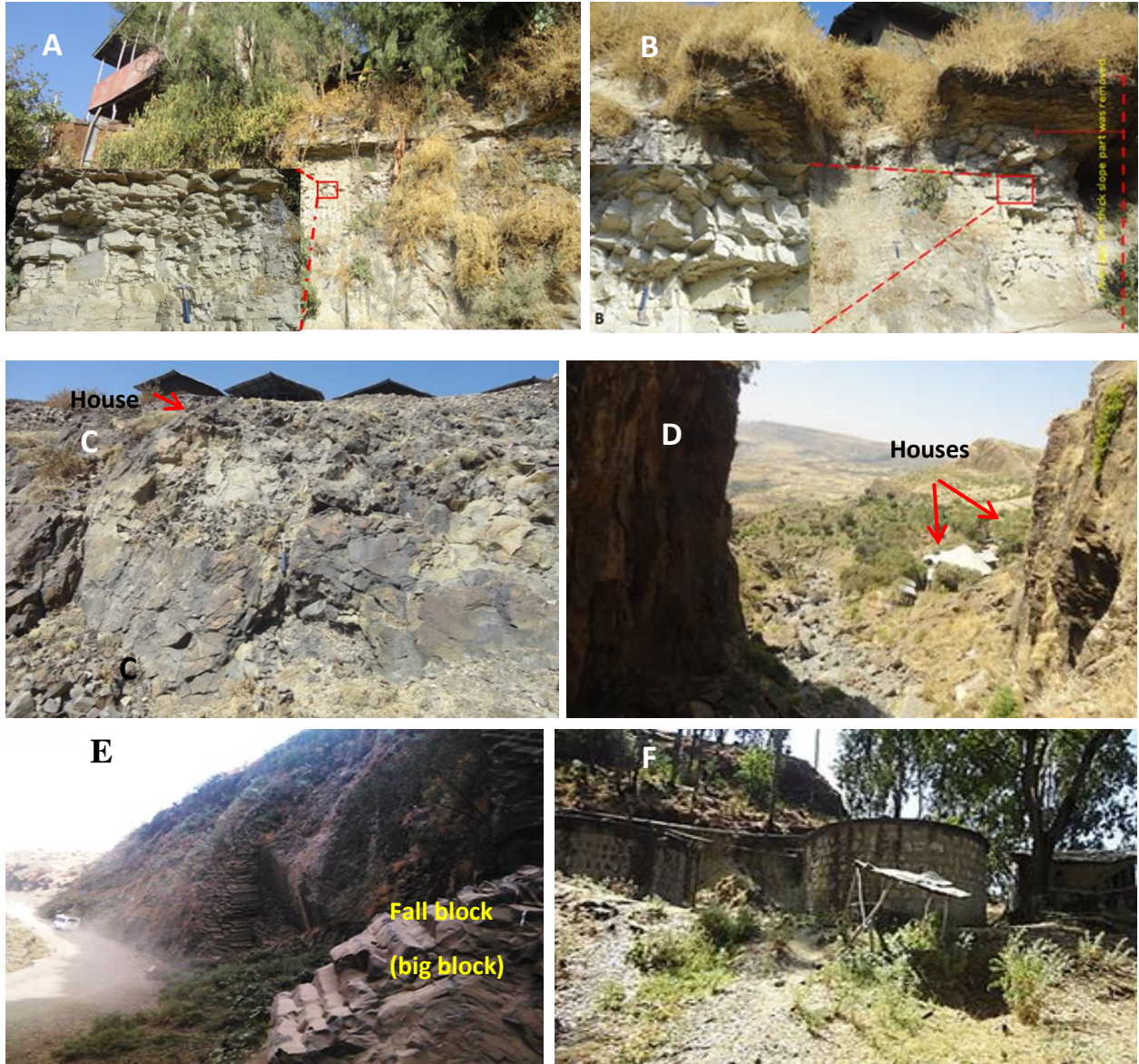
Plate 2.6 slope failure problems in the study area :A and B shows problems on G+1 Buildings constructed at the top of unstable chert slope located at the center of Alem ketema (10°03'21.6" northing and 038°59'44.9" easting); (C) Houses constructed at the top of the valley (D) Houses constructed at the toe of the steep slope (E) Road side problems (Alem ketema to meranya road side exposure) (F) Water tanker constructed at the toe of the slope
