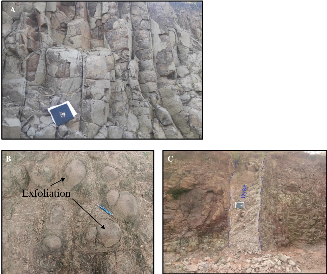
Fig. 3.3: Outcrop photos of Lower basalt. (A) vertical to sub-vertical joints in Lower basalt; (B) Exfoliation weathering on the sparsely porphyritic basalt; and (D) Northeast trending dyke of aphanitic basalt cutting across the sparsely porphyritic basalt.
