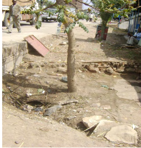
Figure,3.12 Drainage closed by solid waste
