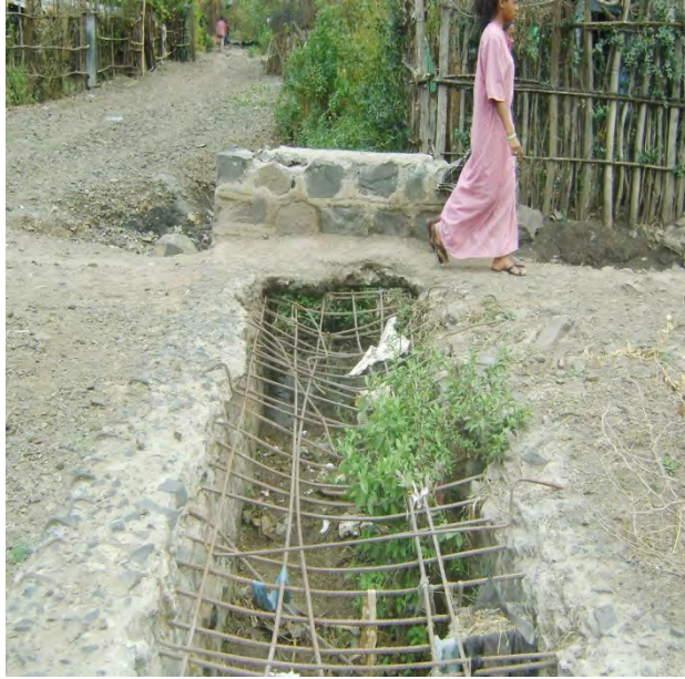
Figure,3.11 Drainage destroyed by overflow
