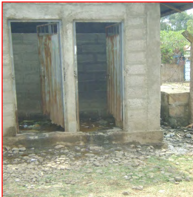
Figure,3.8 Dirty public toilet & Farso house near the toilet.
