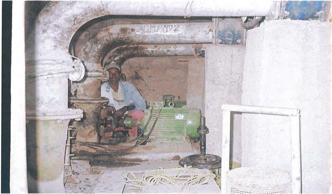
Figure 8: The pumps and the pump operator
