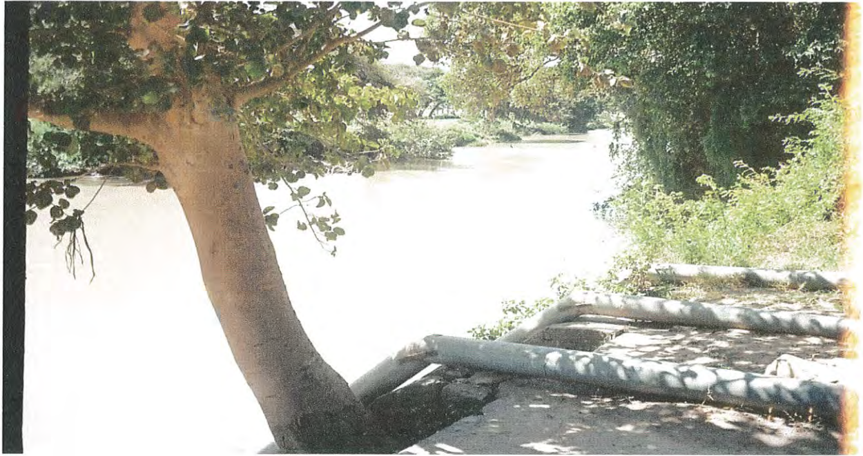
Figure 4: Suction pipes and the Awash River which is the source of water for the project
