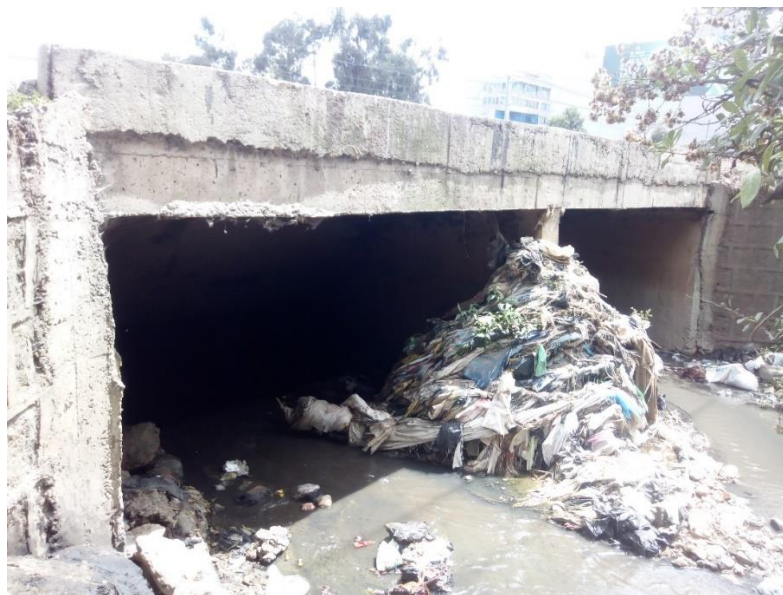
Figure 4.15: Culvert with growing heap of municipal solid wastes around the pier
