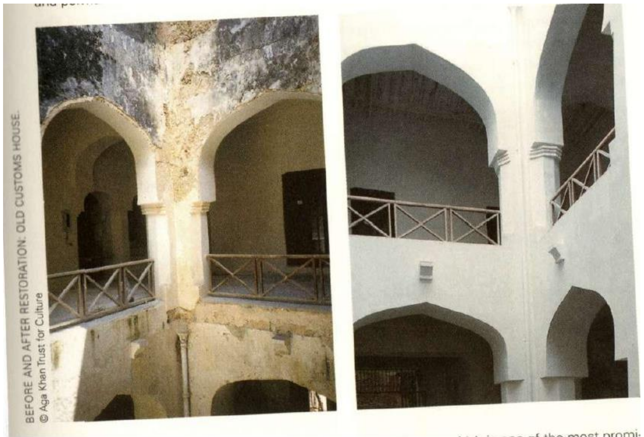
Figure 3-27 A building after Restoration with Lime, from Battle, Melin, and Forsman 2007
