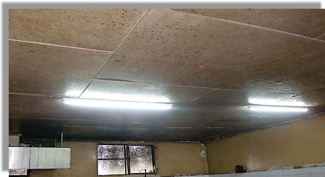
Picture 9:Moisture in Ceiling due to improper installation of ventilation system at Alert Hospital kitchen.
