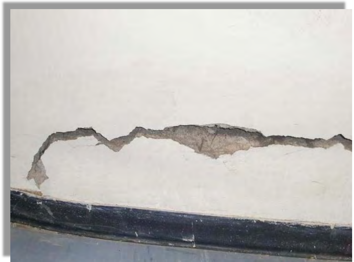
Picture 6 :Crack on wall due to poor design and construction.
