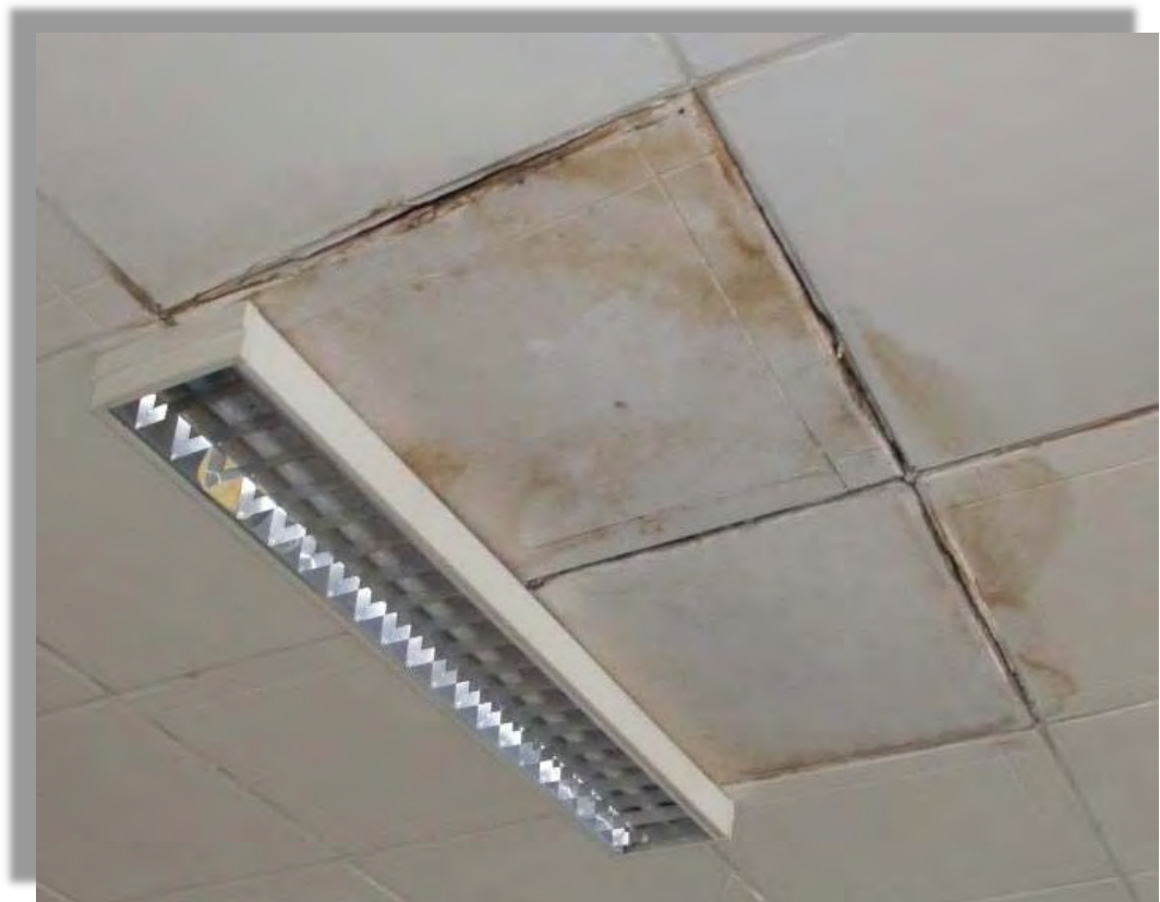
Picture 3 :Moisture in ceiling of patient's bed room due to a leakage from the roof.
