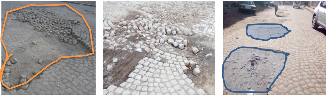
Figure: 4. 59 : degraded Cobblestone roads in the study areas Source: captured by the researcher, 2017
