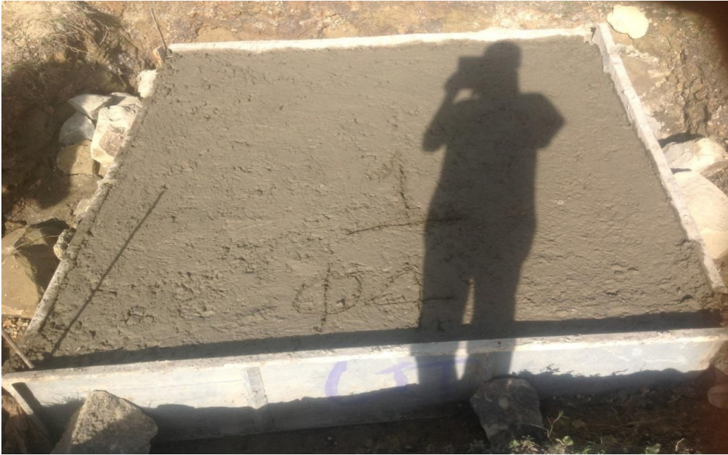
Figure 7 Fresh Concrete Cast of Sample #1(6cm thick concrete and \phi 4 wire mesh)
