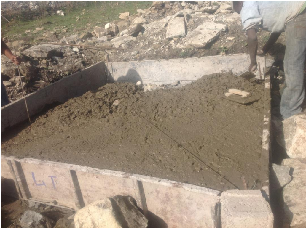
Figure 8 Fresh Concrete Cast of Sample #2 (6cm thick concrete and \phi 2.5 wire mesh)
