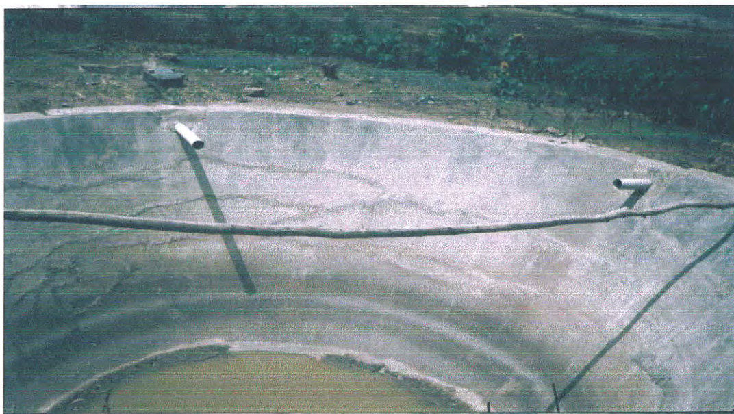
Picture 5.5: Cracks in the RWH Structure in Abahilme Kebele, March 2005
