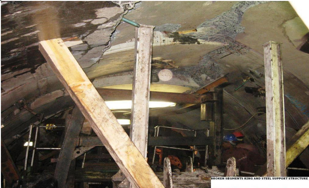
Figure 15 Lining segments moved and severely damaged [4].
