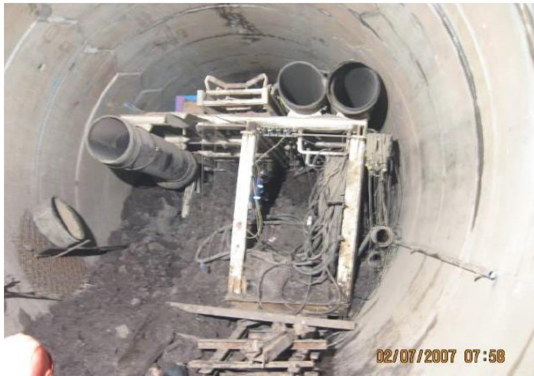
Figure 18 Consolidated mud filling the Power Tunnel [4]
