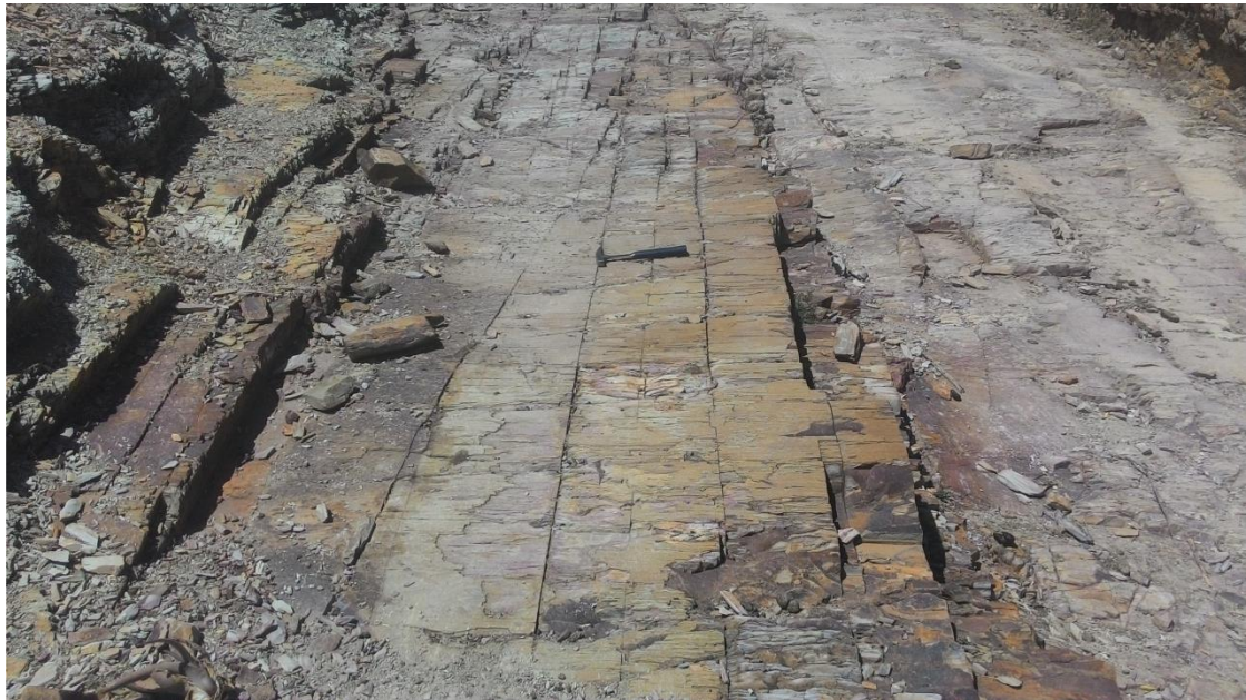
Fig.5.4: Systematic joint sets in lower slate unit. This systematic joint has N-S trending (0505000E:1535439N).
