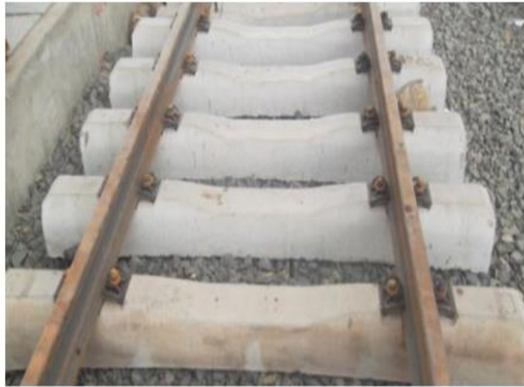
Figure 3.7: Addis Ababa LRT sleeper.
