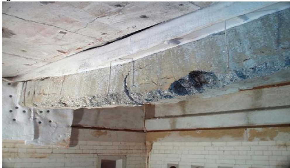
Fig. 4.47: A typical girder under crack
