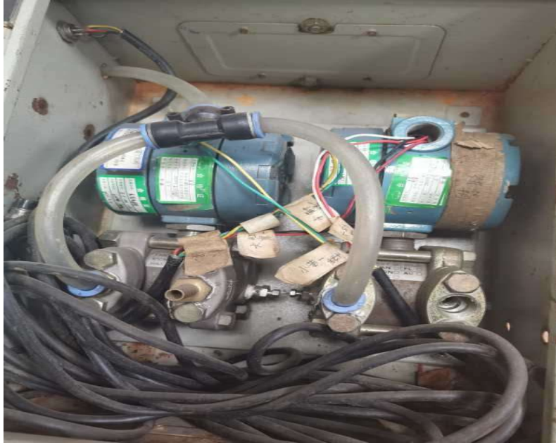
Figure 5-11: Differential pressure transmitter used to measure air pressure difference
