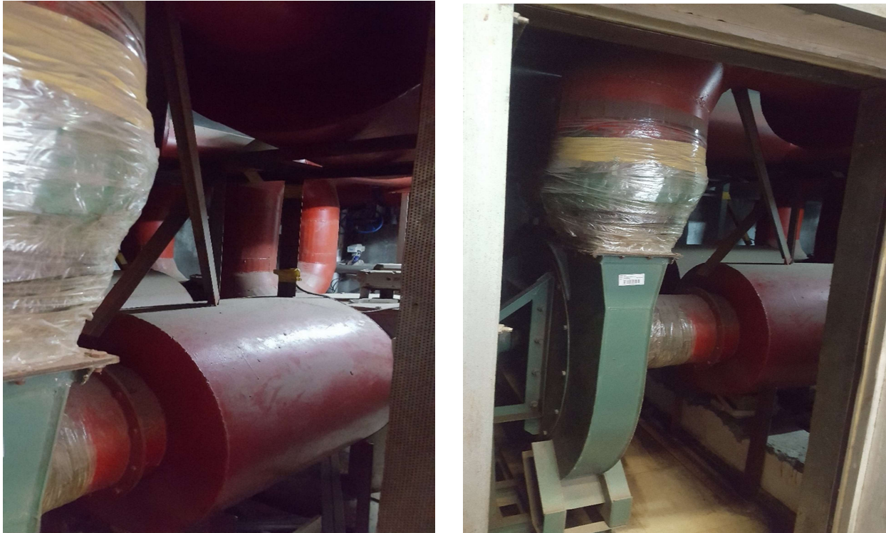
Figure 5-9: Air supply and exhaust machine
