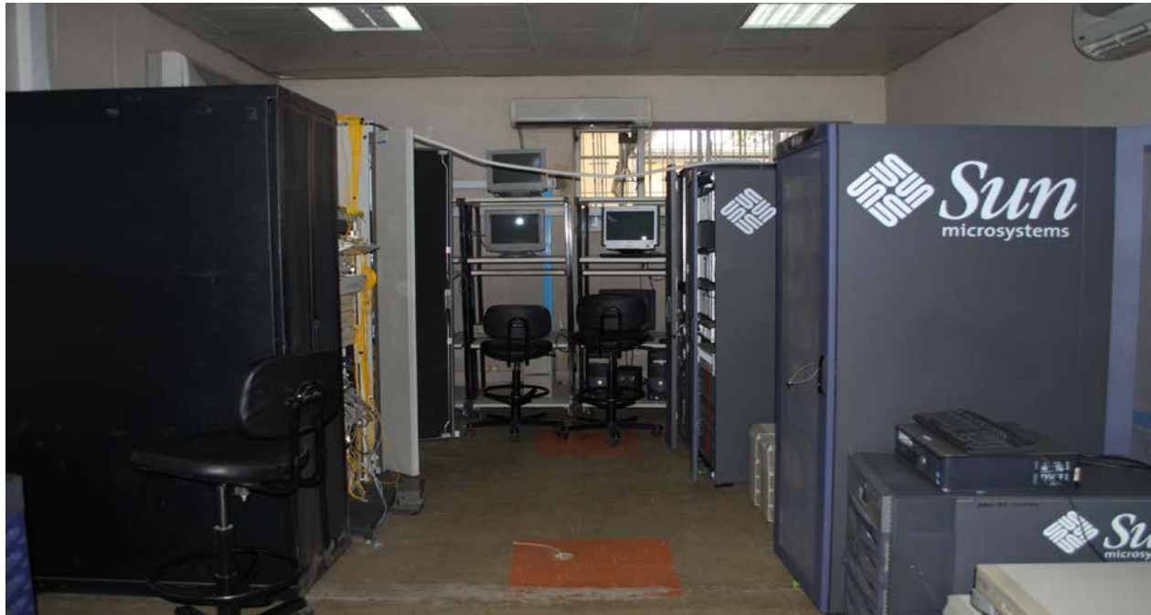
Figure 3.2: AAU Data Center
