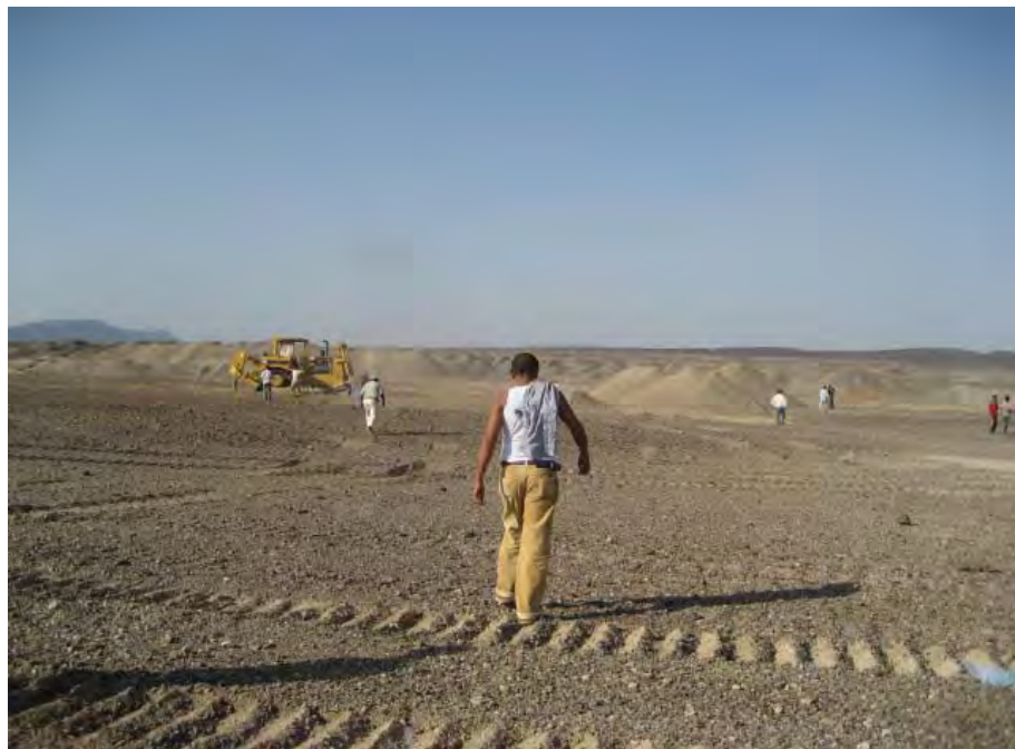
Figure3.2: Material site: a) borrow area for clay core, and b) for sandy gravel shell.
