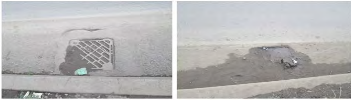
Figure 20: Blocked inlets by the side of roads
