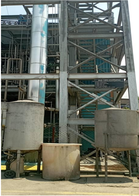
(a) Ethanol/alcohol production plant
