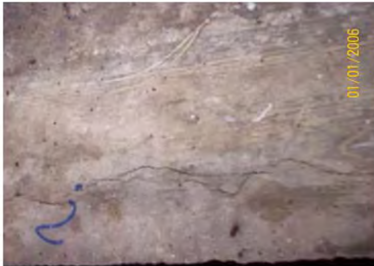
Figure 5.4 Cracks That were Observed during Curing Period in 4.5% Beam Specimen
