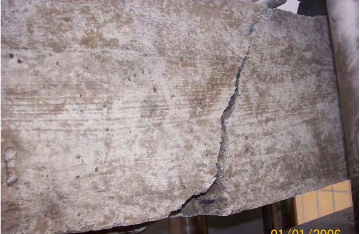
Figure 4.12 Failure pattern for F-untreated, 3.5-9
