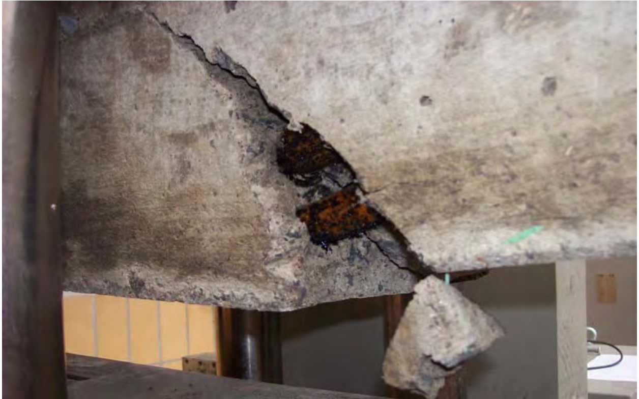
Figure 4.6 Failure pattern for F-treated, 2.5-3
