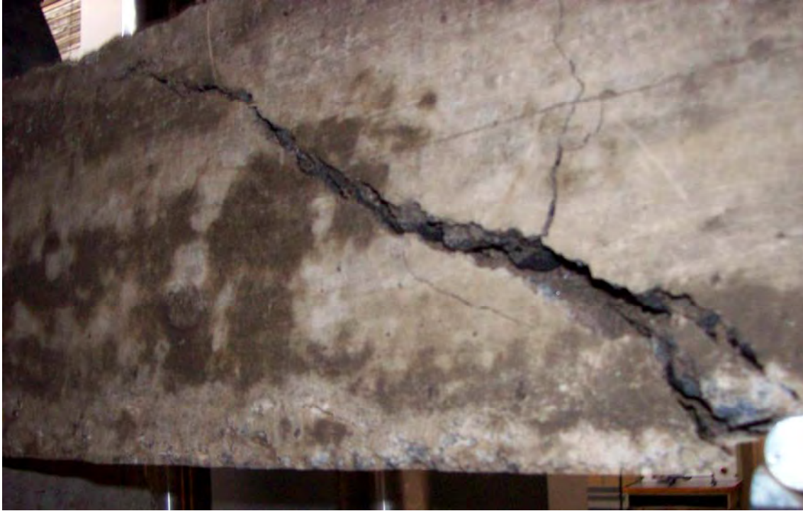
Figure 4.7 Failure pattern for F-untreated, 2.5-4
